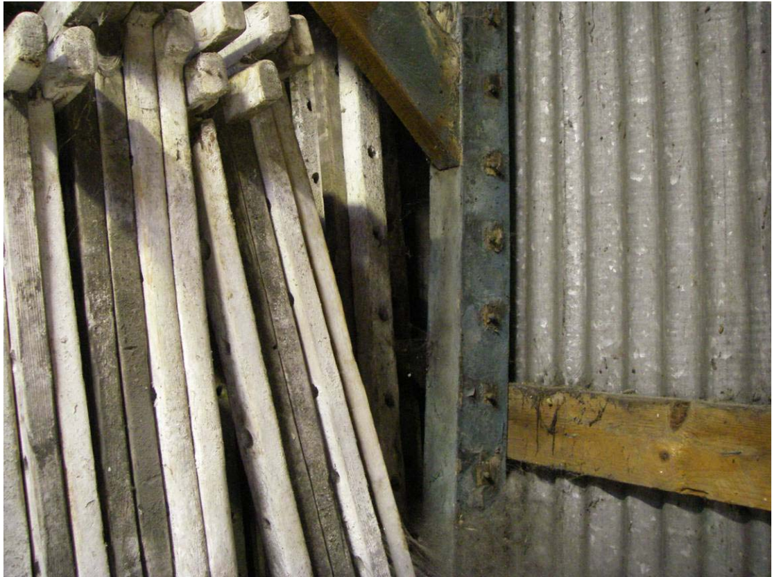
Plate 27: First floor to show position of former louvers (Photograph taken by Christiane Meckseper)
