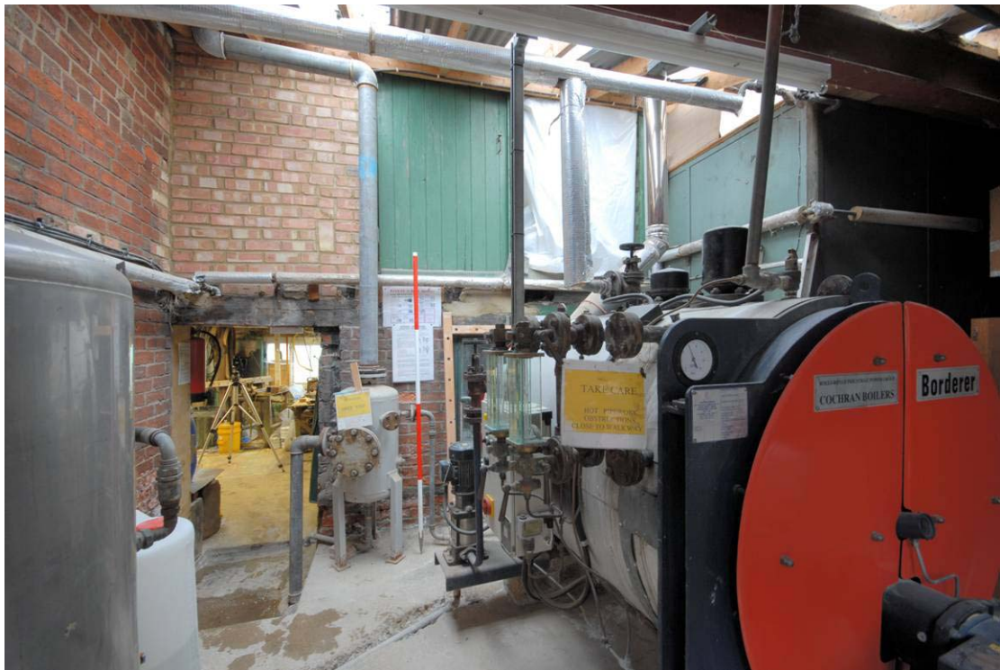
Plate 20: Boiler room G
