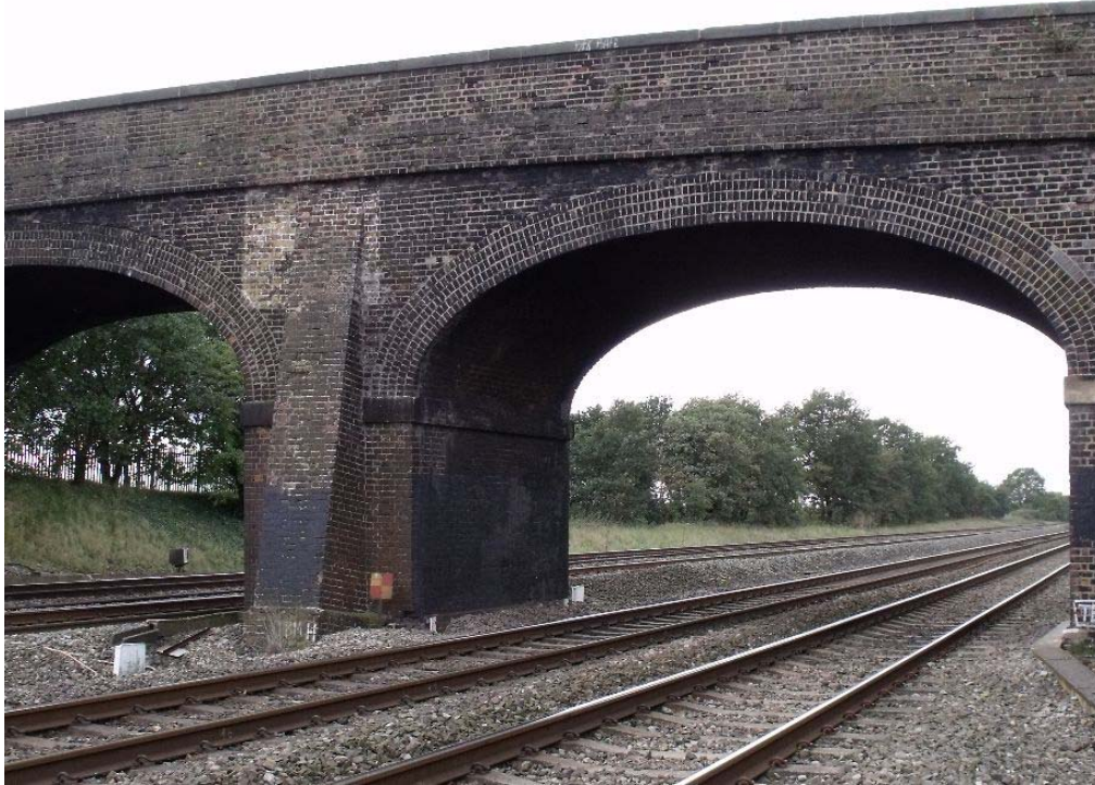
Figure 6: Dog Kennel Bridge east facing elevation. Northern extension arch and central buttress with changeover in brickwork. (Photo: Total Surveys Ltd.)
