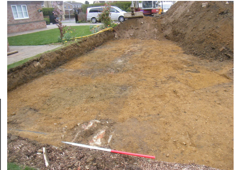
East half of PDA showing foundations and drains. Looking SSE. Scale 1m
