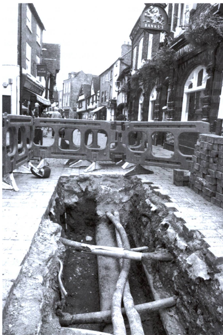
Fig. 58: Friar Street gas main
