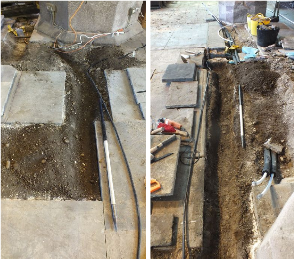
Plate 9 (left): South end of Trench E during excavation, viewed from the north
