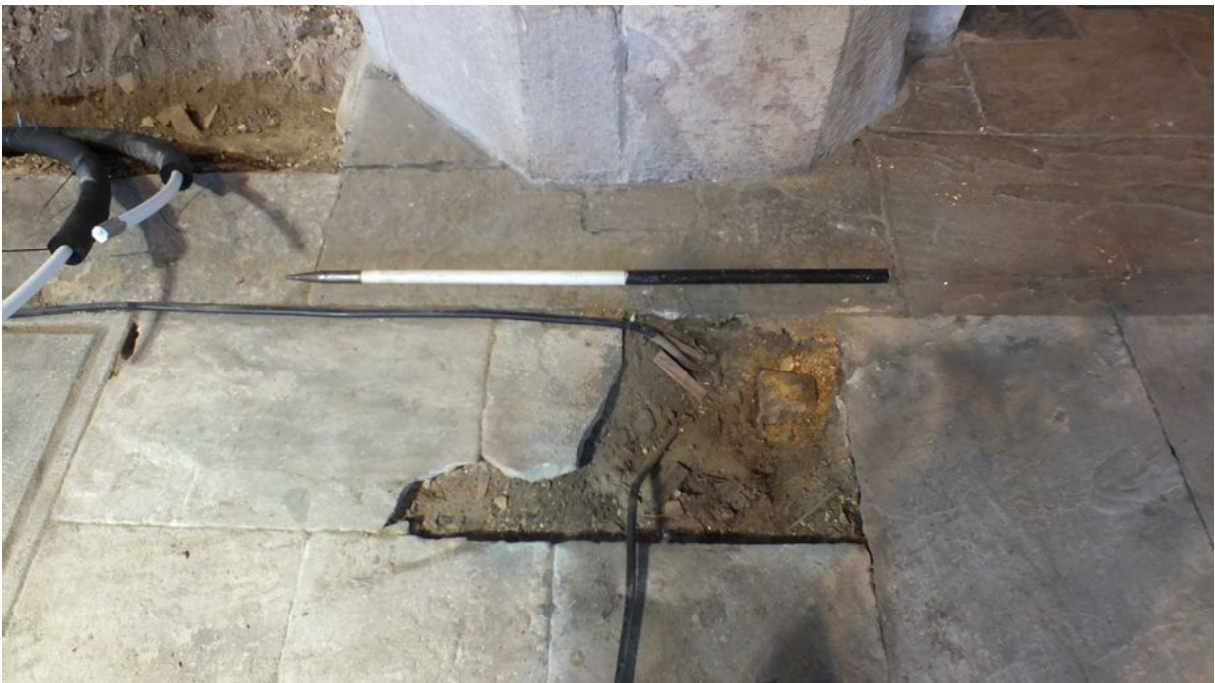
Plate 8: Existing hole prior to excavation of Trench E, viewed from the south
