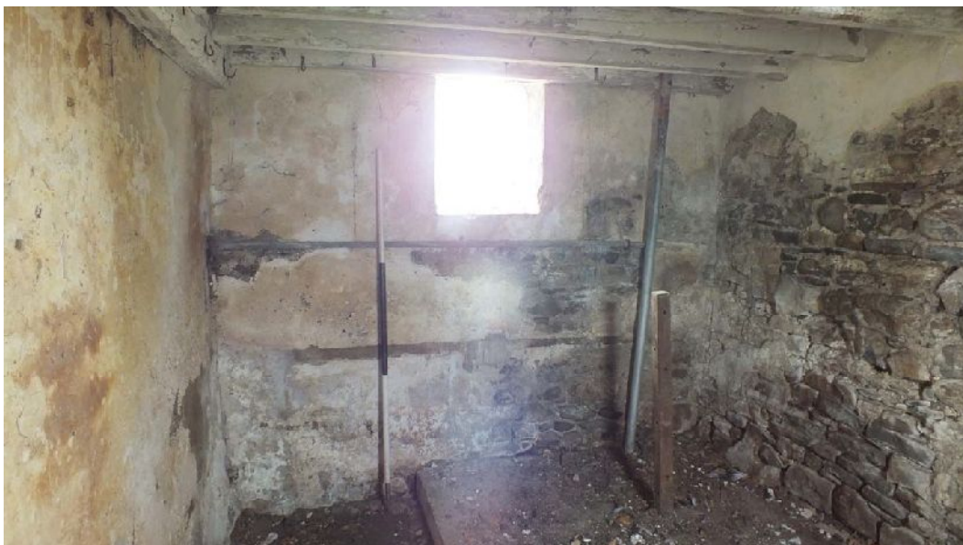
Plate 47: South elevation of lower floor Room 2 of Building B, from the north
