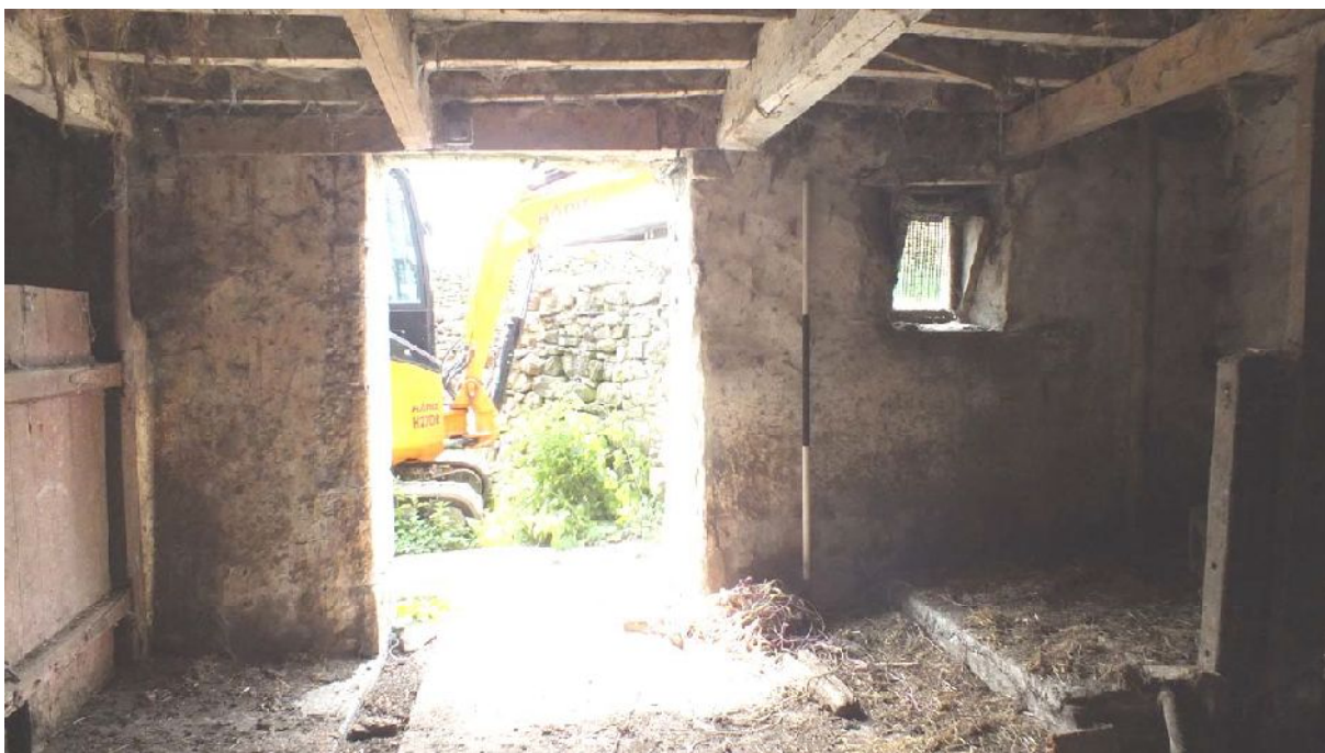
Plate 28: South elevation doorway and window in lower floor Room 2 of Building A, from the north
