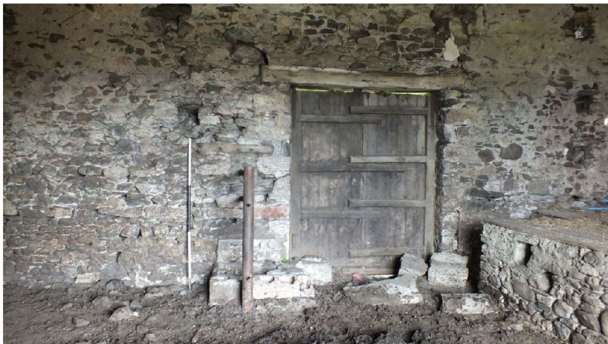
Plate 32: North elevation door in upper floor of Building A, from the south
