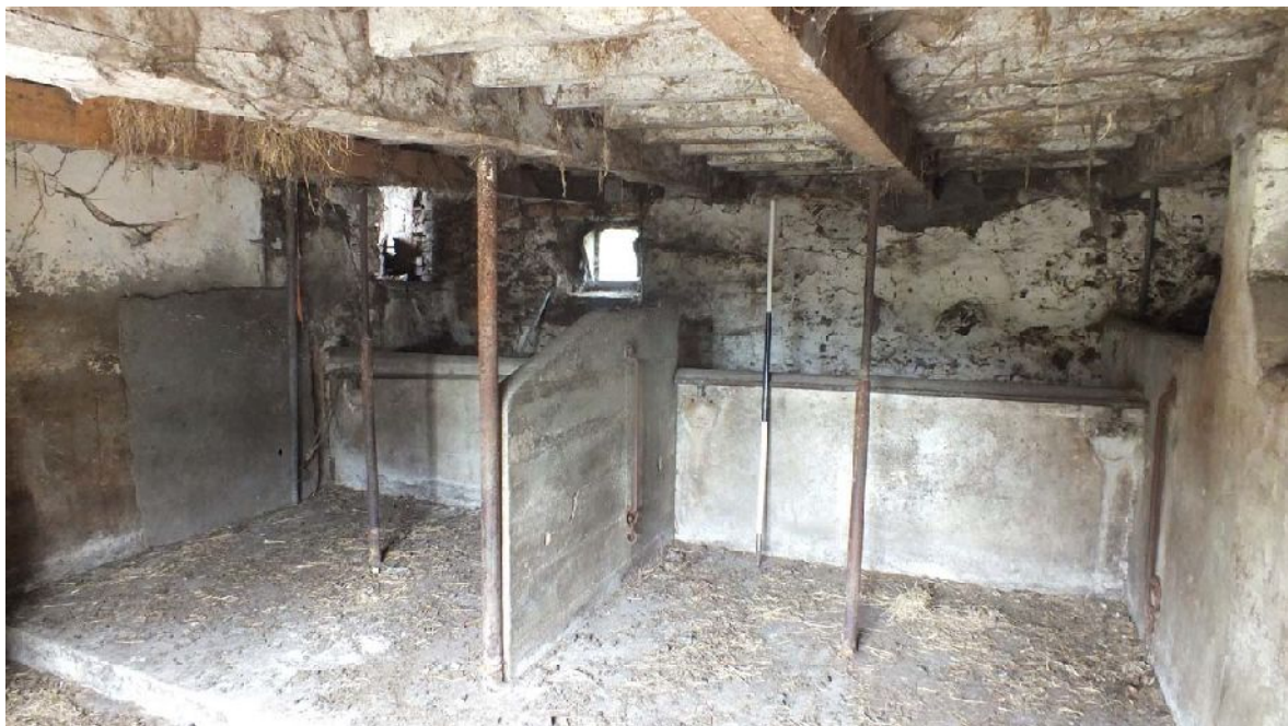
Plate 24: Stalls on the north side of Building A, lower floor Room 2, from the south-east
