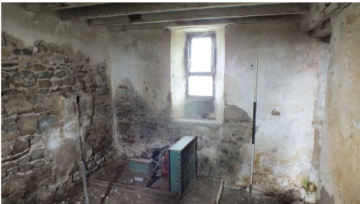
Plate 45: North elevation of lower floor Room 2 of Building B, from the south
