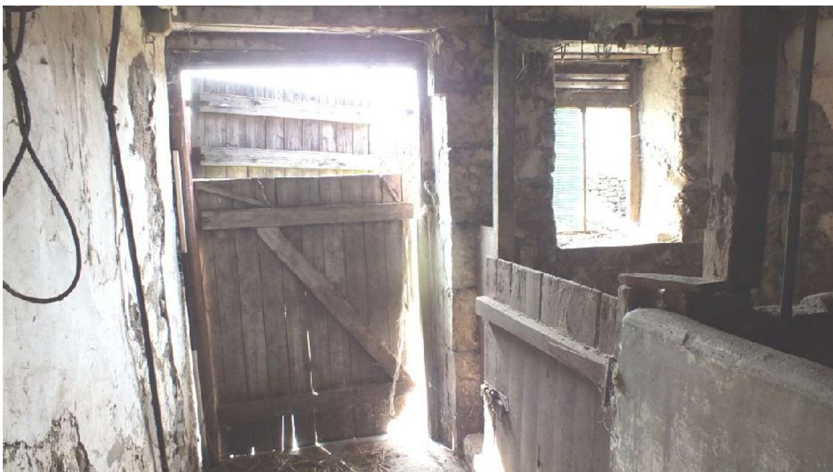
Plate 22: Door and window in lower floor Room 1 of Building A, from the north
