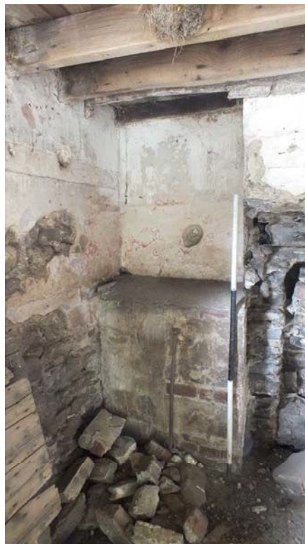
Plate 44: Added bricks on south side of west elevation of lower floor Room 1 of Building B, from the north-east
