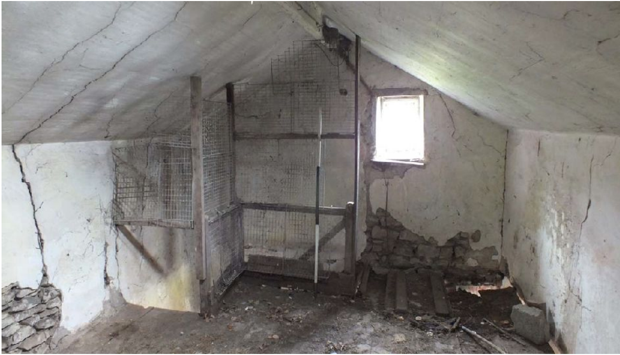
Plate 49: East end of first floor Room 1 of Building B, from the west
