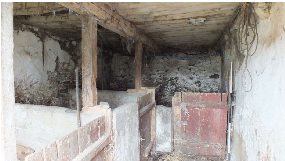
Plate 21: Stalls and ceiling in lower floor Room 1 of Building A, from the south
