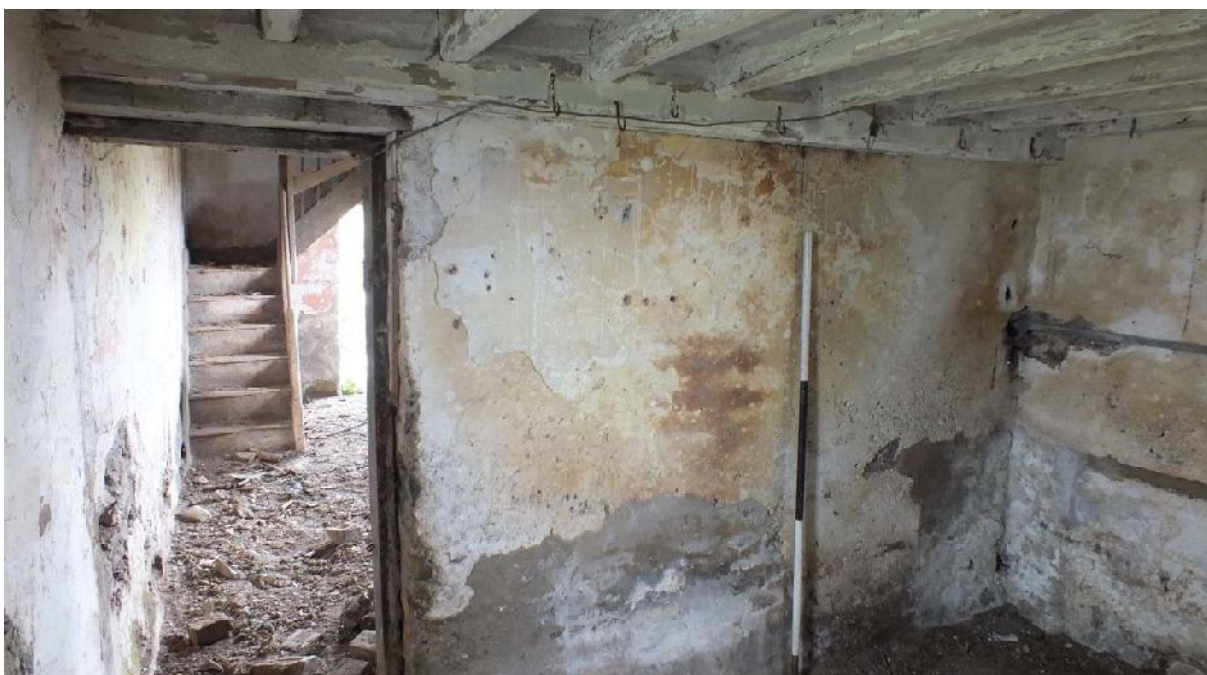
Plate 46: East elevation of lower floor Room 2 of Building B, from the west
