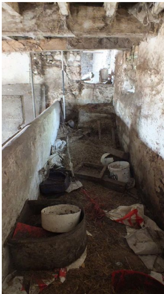
Plate 29: West elevation door in lower floor Room 2 of Building A, from the east
