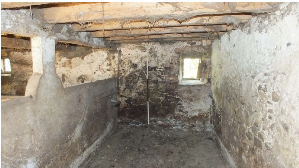
Plate 27: Window on the east side of the north elevation in lower floor of Room 2 of Building A, from the south
