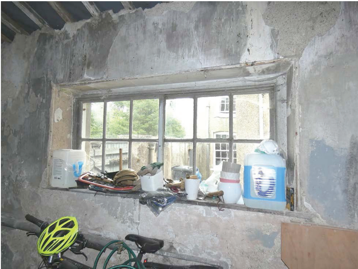
Plate 23: Horizontal sliding sash window in the east elevation of Room G1, viewed from the south-west
