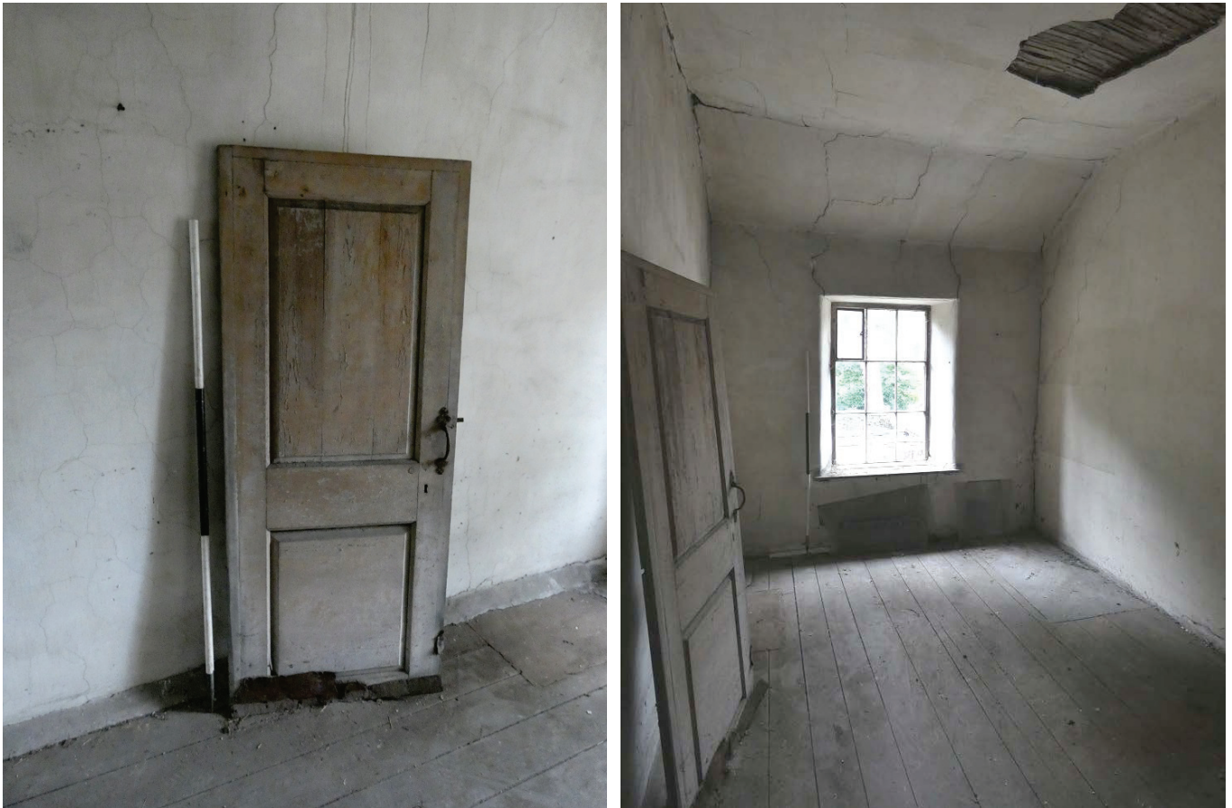
Plate 53 (left): Loose door in Room F3, viewed from the north-west
