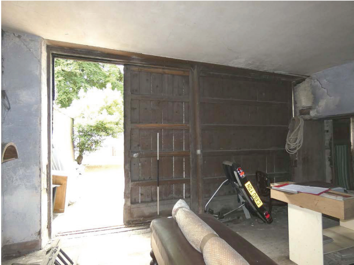
Plate 33: Sliding wagon doorway in the south elevation of Room G4, viewed from the north
