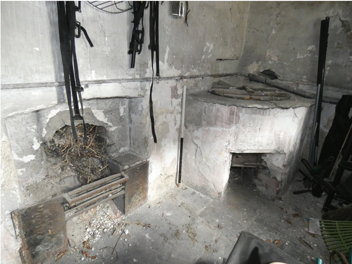
Plate 24: Hearth and copper on the west side of Room G1, viewed from the south-east
