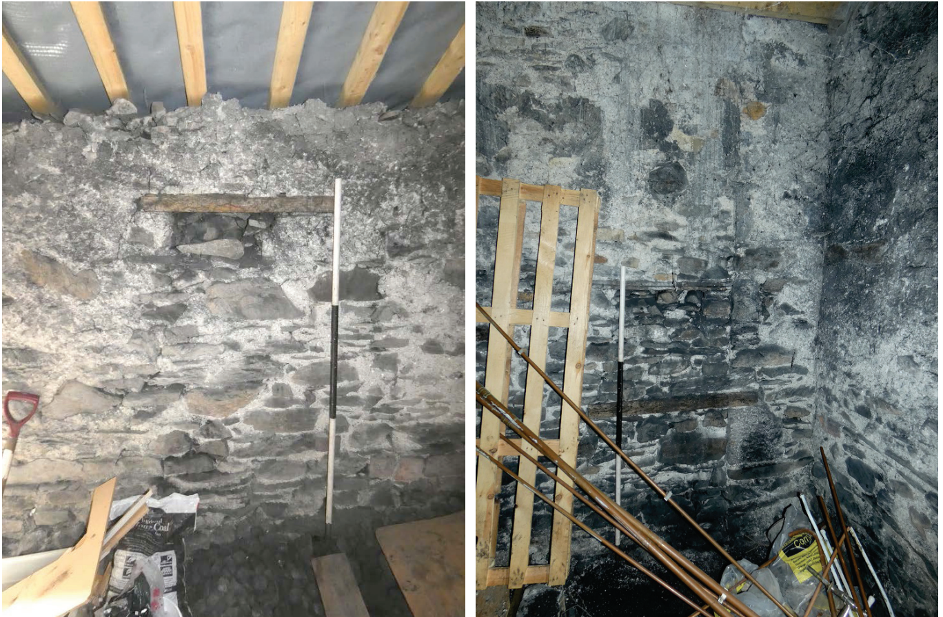
Plate 29 (left): Small alcove in the east elevation of Room G3, viewed from the west
