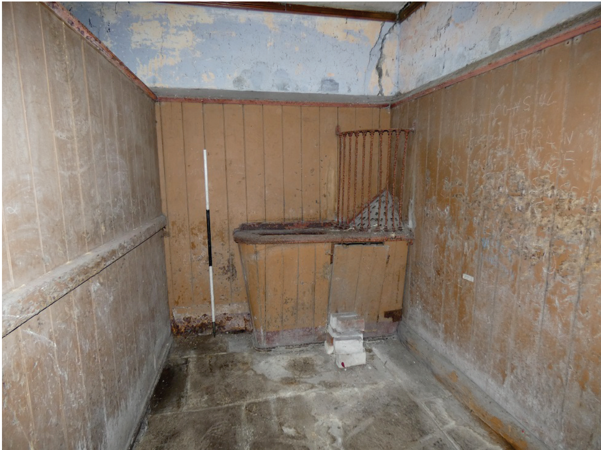
Plate 39: Detail of manager and feed trough in the northern stall in Room G6, viewed from the east
