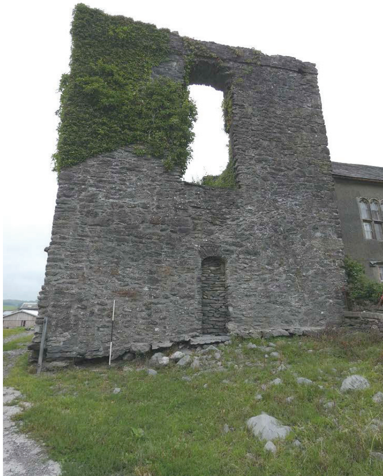
Plate 5: The site prior to excavation showing the extent of the south-west wall of the tower
