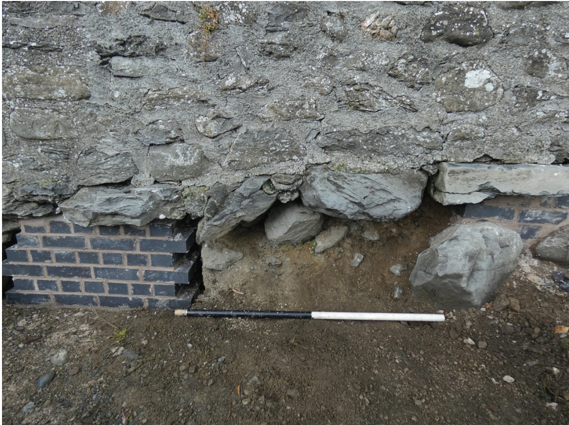
Plate 8: Excavation north-west of the alcove showing exposed boulders in 101, with new brickwork showing on either side
