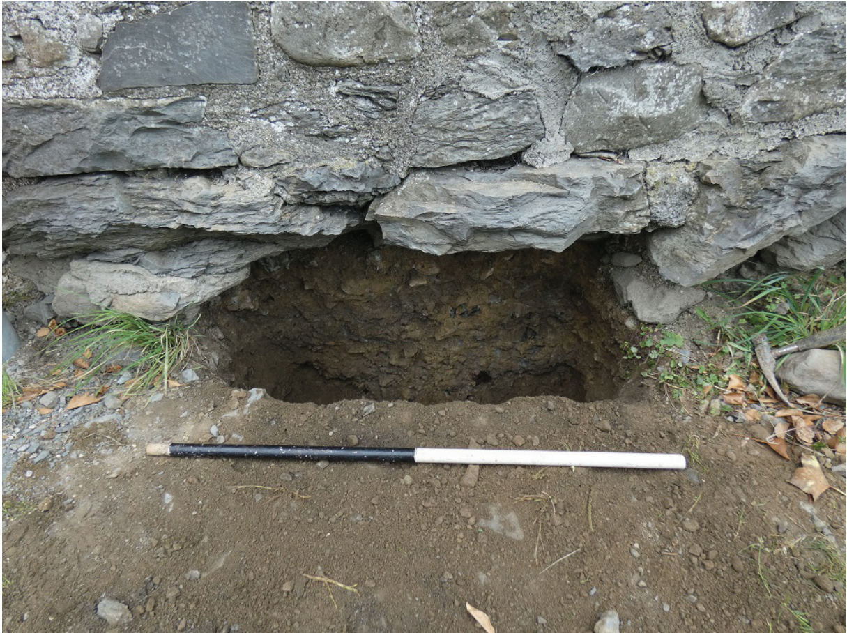
Plate 7: Excavation to a depth of 0.5m on the north-west side of the wall
