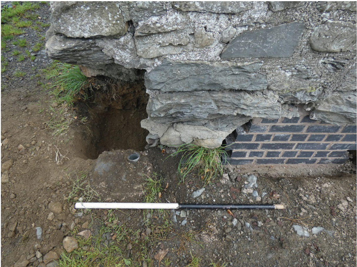
Plate 10: Excavation beyond the west corner showing deposits exposed and areas of previous disturbance, with newly inserted brickwork visible
