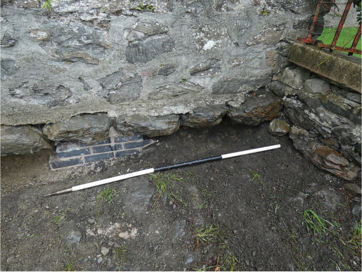
Plate 11: Deposit 101 exposed at the south-east end of the wall and the adjoining boundary wall, with newly inserted brickwork visible
