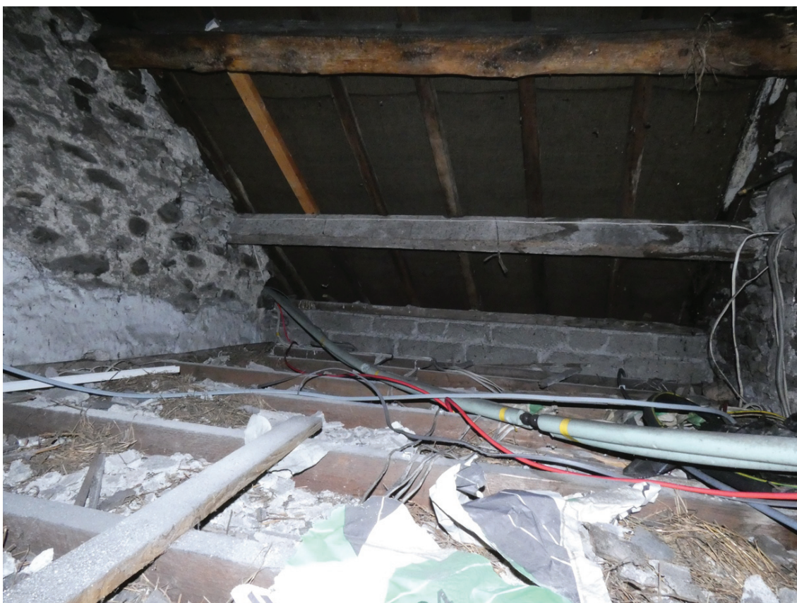
Plate 63: Concrete block rebuild to the east side of G7, viewed from inside the roof space
