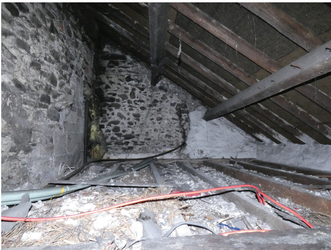
Plate 62: General view of the south end of the roof space above G7
