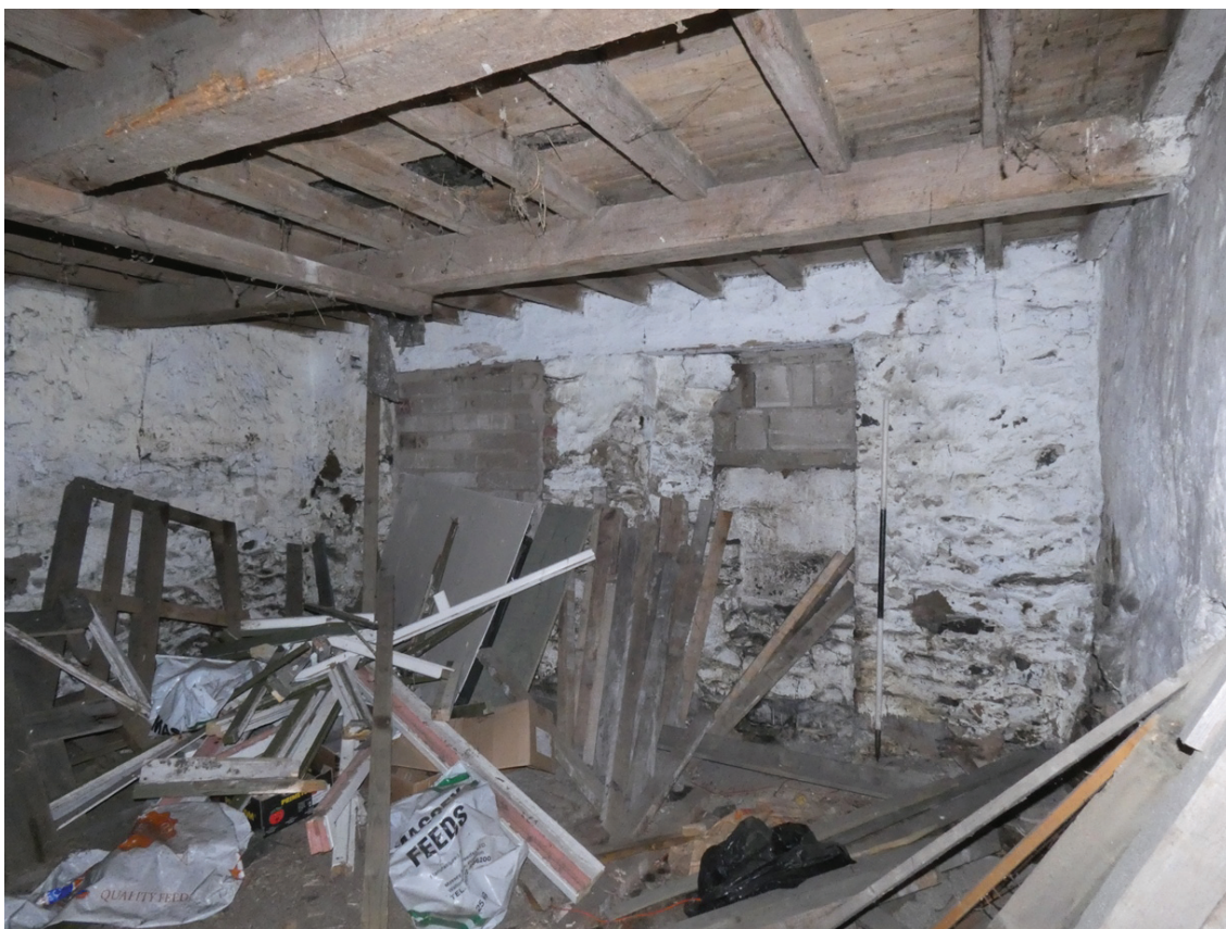
Plate 27: Blocked doors at the north end of G1
