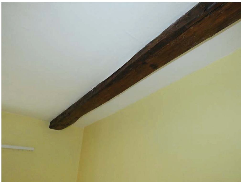
Plate 29: Beam along the south side of the northern bedroom, viewed from the north-west
