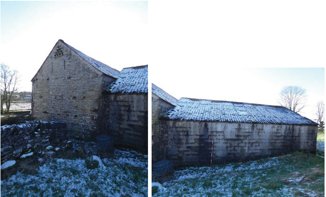
Plate 8 (left): The gable end of the barn forming the main part of the north external elevation, viewed from the north-west
