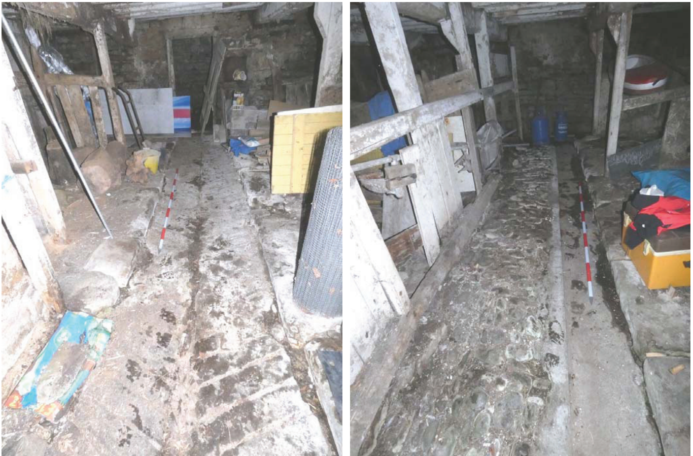
Plate 29 (left): Dung channel in the floor on the south side of Room L3, viewed from the east
