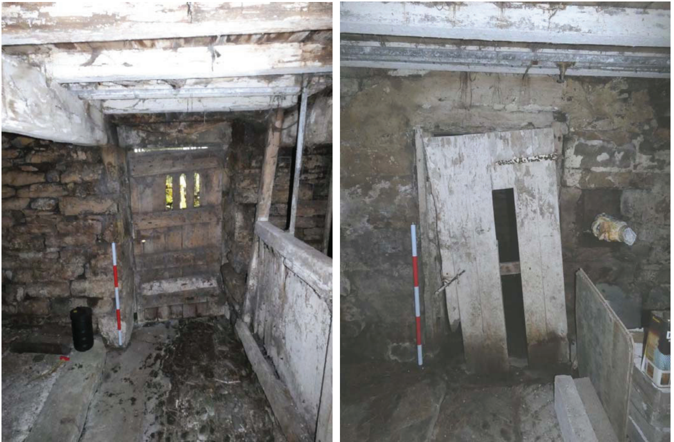
Plate 35 (left): Door in the north side of the east elevation of Room L3, viewed from the west
