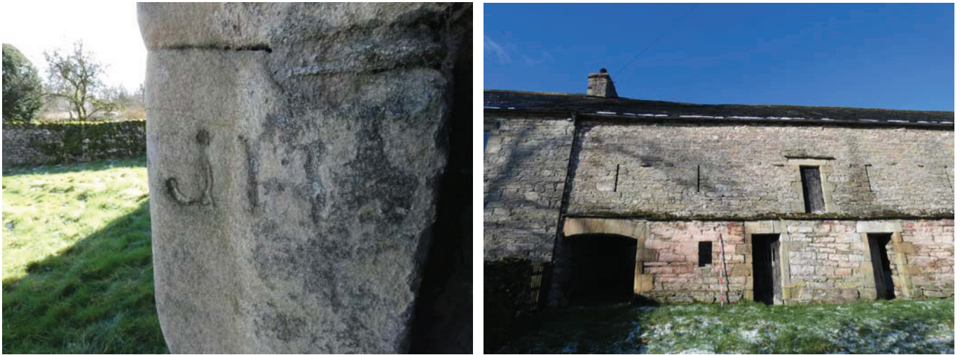
Plate 13 (left): Graffiti on the southern jamb of the southernmost doorway in the east external elevation, viewed from the north
