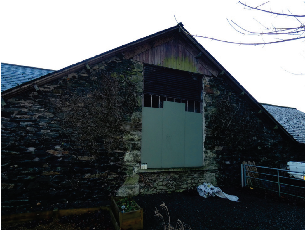
Plate 16: The central gable in the west external elevation of the building, viewed from the west
