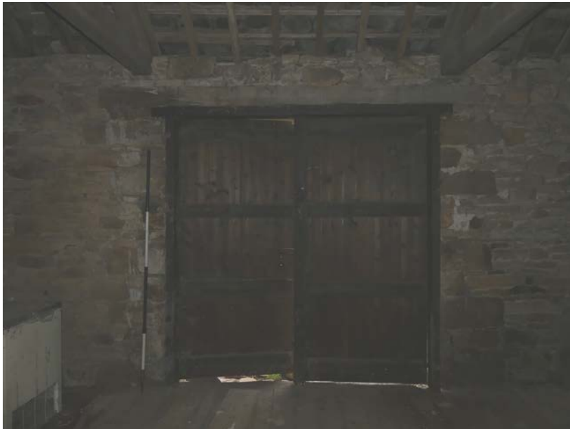
Plate 26: Wagon doorway in the west elevation of upper ground floor Room 1, viewed from the east
