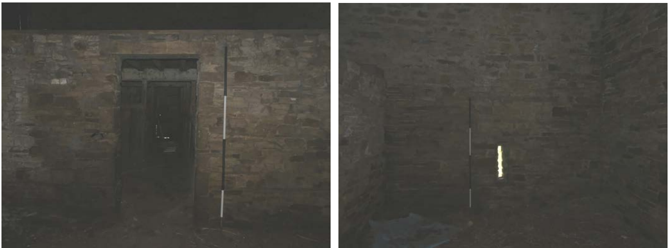
Plate 38 (left): Doorway in the north elevation of lower ground floor Room 2, viewed from the south
