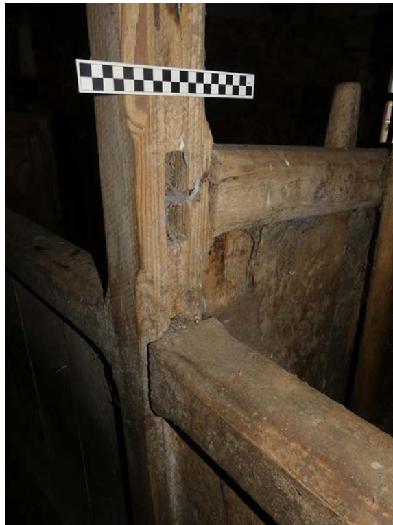
Plate 31: Altered section of the eastern stalls in lower ground floor Room 1, viewed from the south-west
