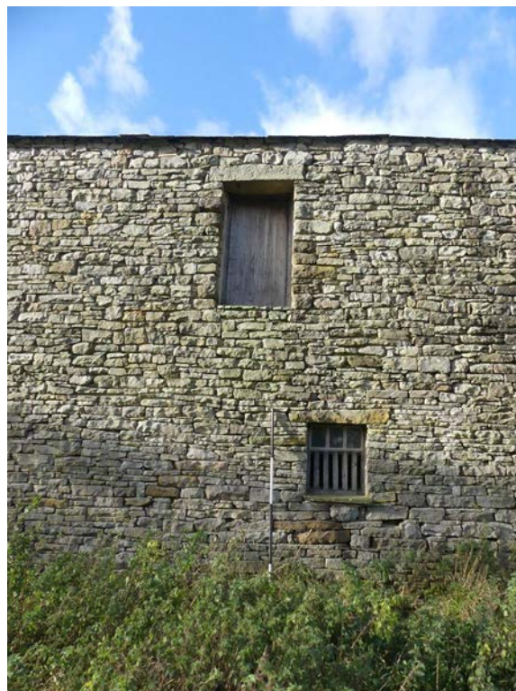
Plate 13: Upper ground floor doorway in the east external elevation, viewed from the east
