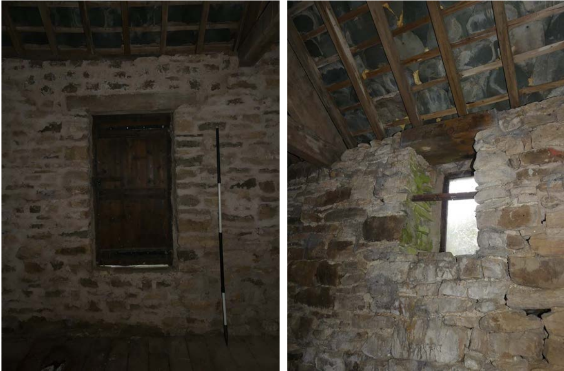
Plate 24 (left): Doorway in the east elevation of upper ground floor Room 1, viewed from the west
