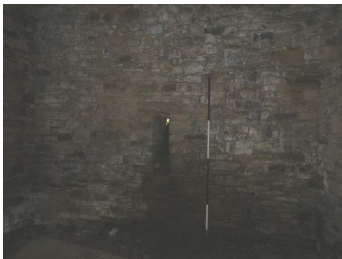
Plate 40: Ventilation slot in the west elevation of lower ground floor Room 2, viewed from the east
