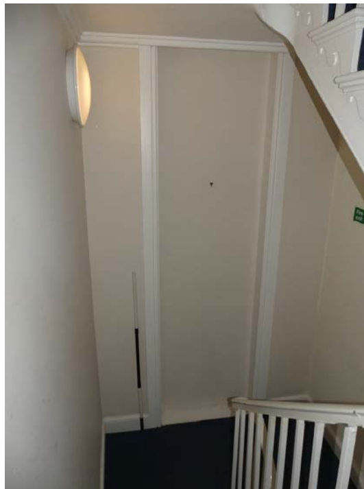
Plate 55: Former window in the west elevation of Room F2, viewed from the east
