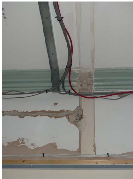
Plate 83: Earlier stud partition scar exposed on the north elevation, viewed from the south
