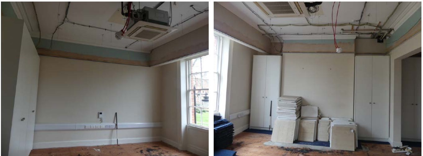
Plate 89 (left): General view of Room F4 following soft stripping, viewed from the south
