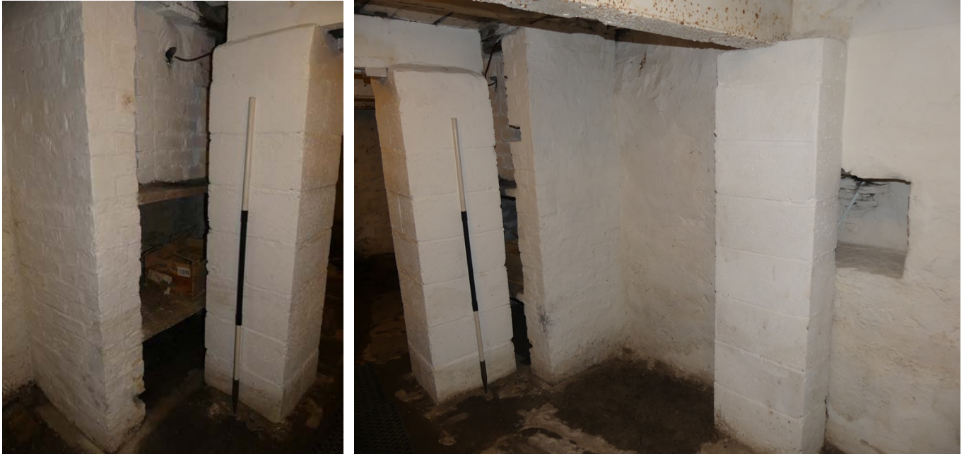
Plate 42 (left): General view of the centre section of the north-west elevation of the basement
