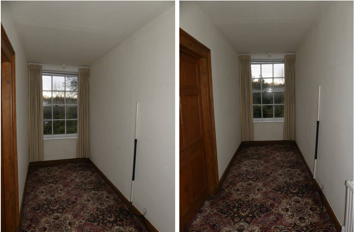
Plate 129 (left): Scar in the north-west elevation of Room F4
