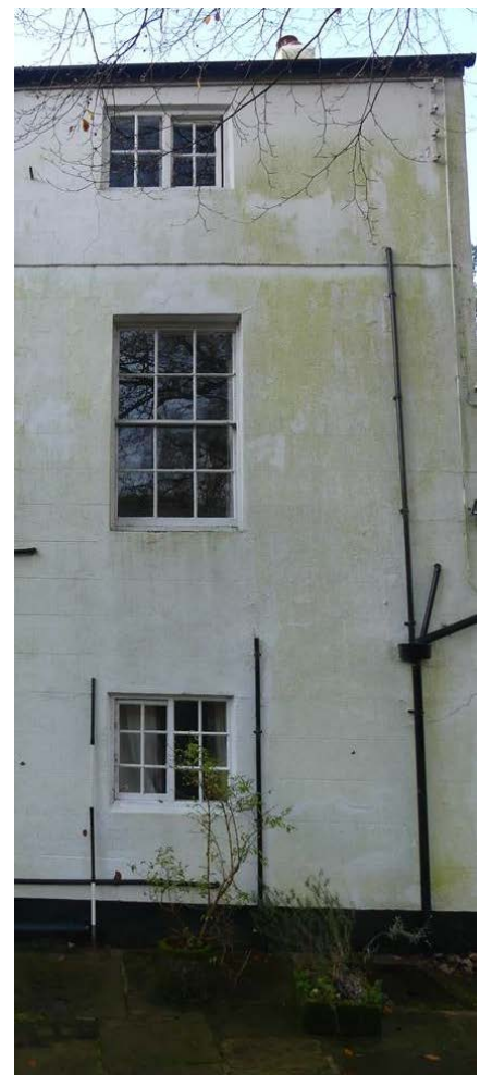
Plate 25 (left): South-east end of the north-east external elevation of the main house
