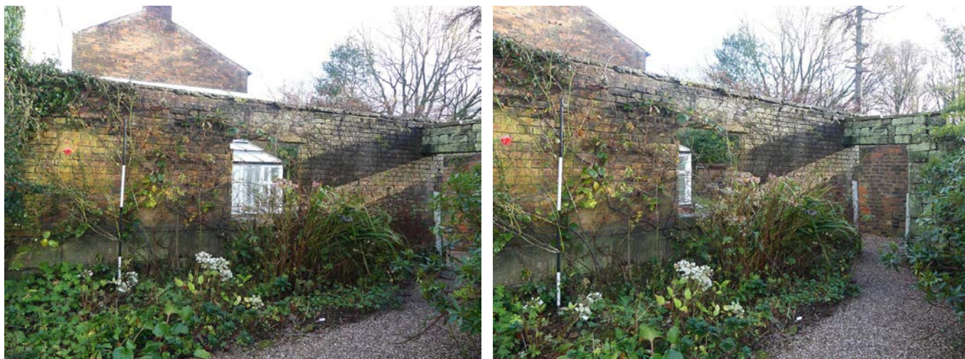
Plate 14 (left): Window in the brick wall to the south-east end of the south-west external elevation
