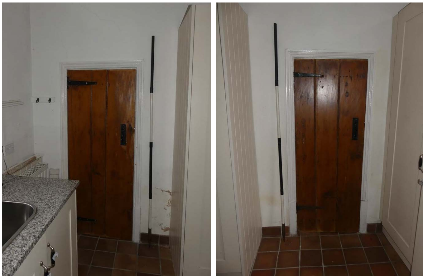
Plate 46 (left): Door to the north-west end of the north-east elevation of Room G1 Plate 47 (right): Door to the south-east end of the north-east elevation of Room G1
