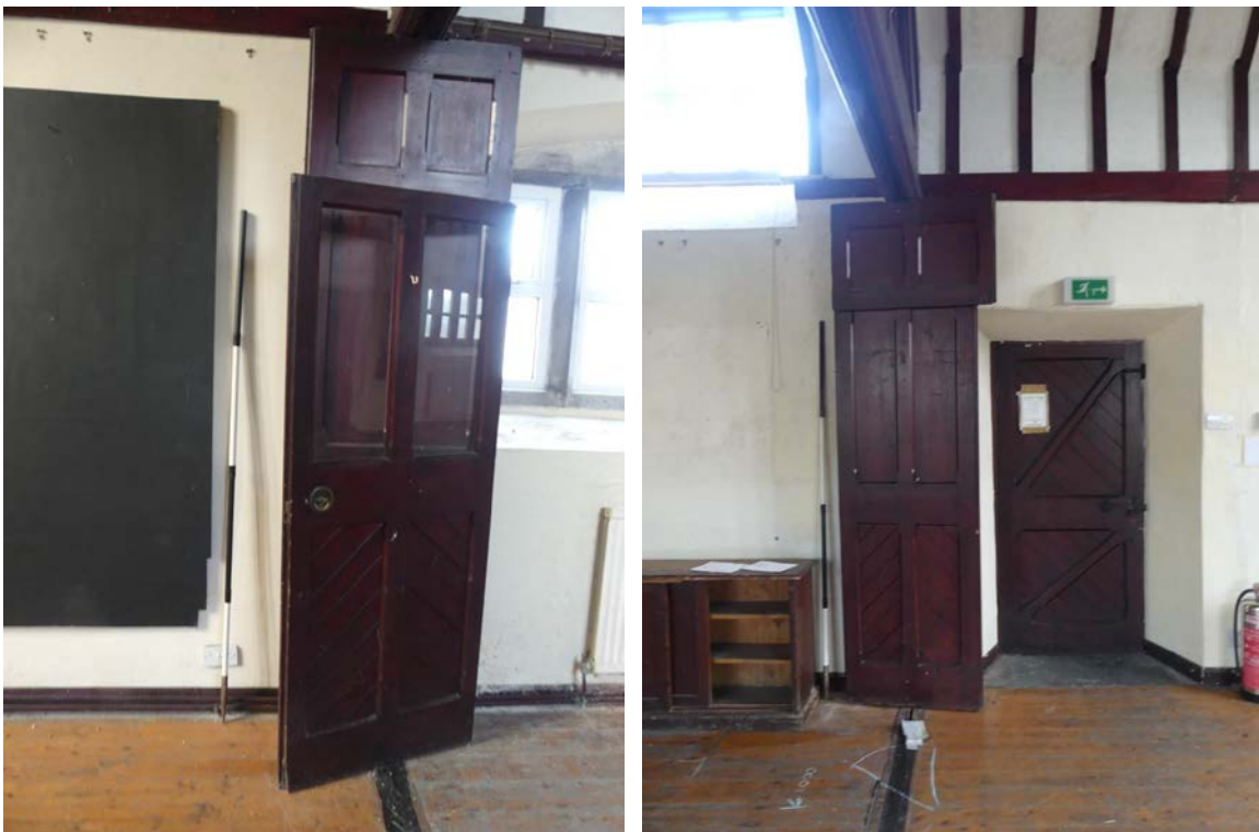
Plate 20 (left): The west side of the folding partition in Room G1, viewed from the east
