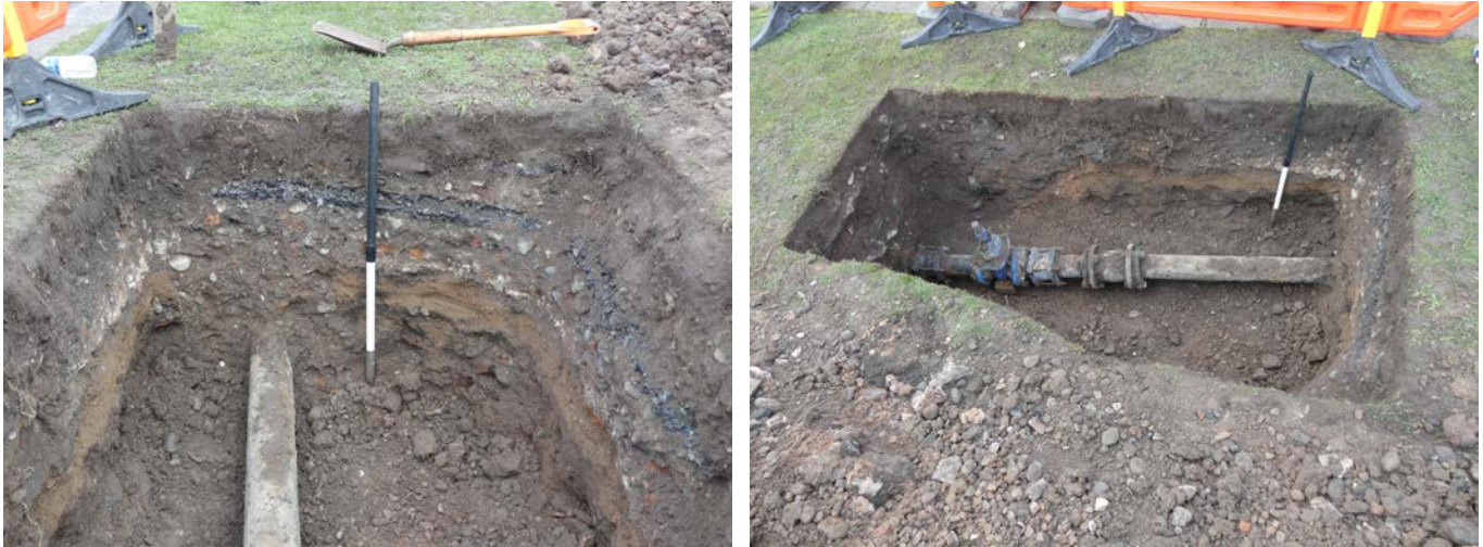
Plate 7: South-east facing section showing deposits 1001, 1003 and 1004, and cut 1007 for the pipe, viewed from the south-east
