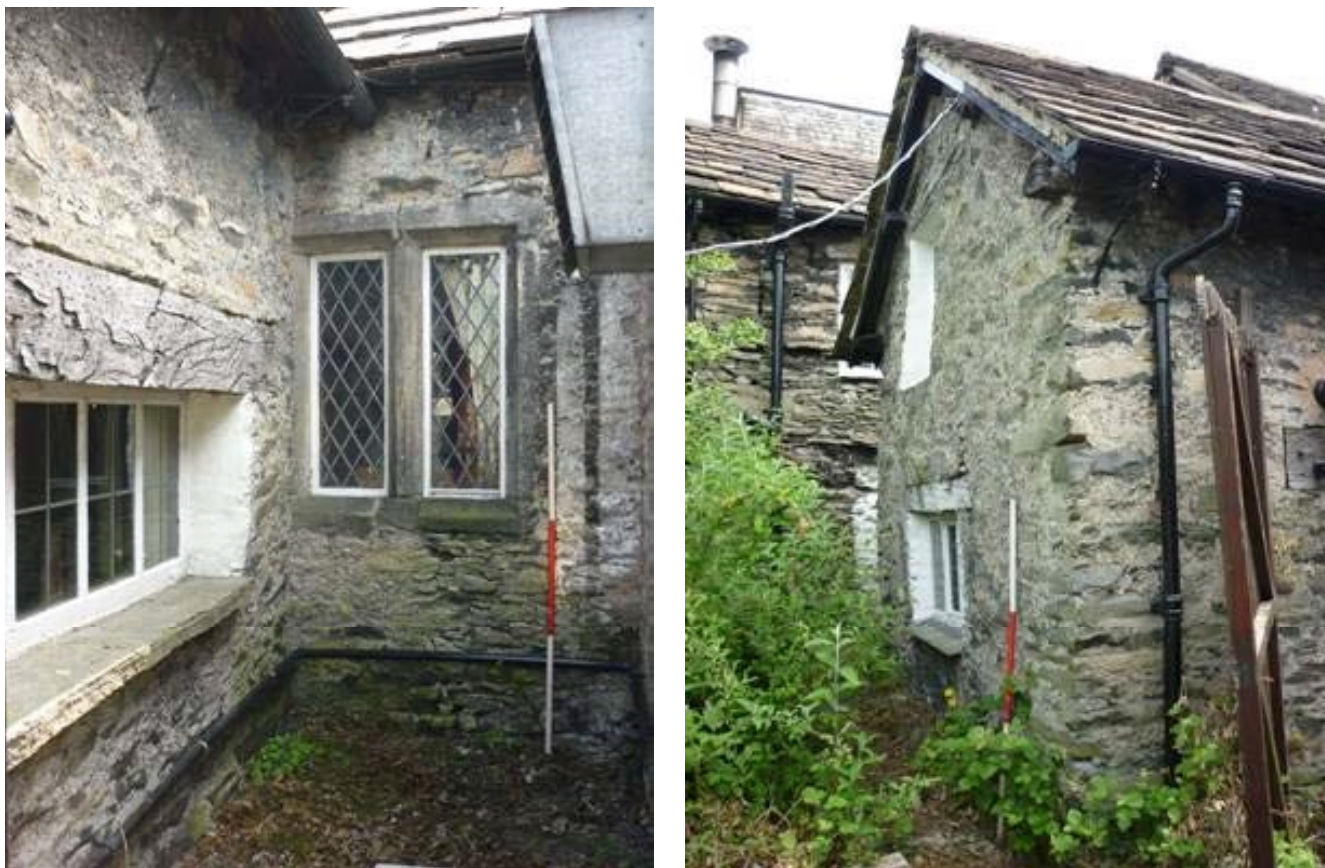
Plate 43 (left): Mullion window between the modern outshut and the extension to the north-east of it Plate 44 (right): North-west end of the smaller of the two extensions at the north-east end of the north-west elevation
