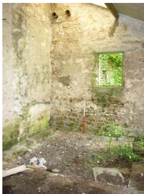
Plate 19 (right): Site 08 - internal view showing the sunken area of floor
