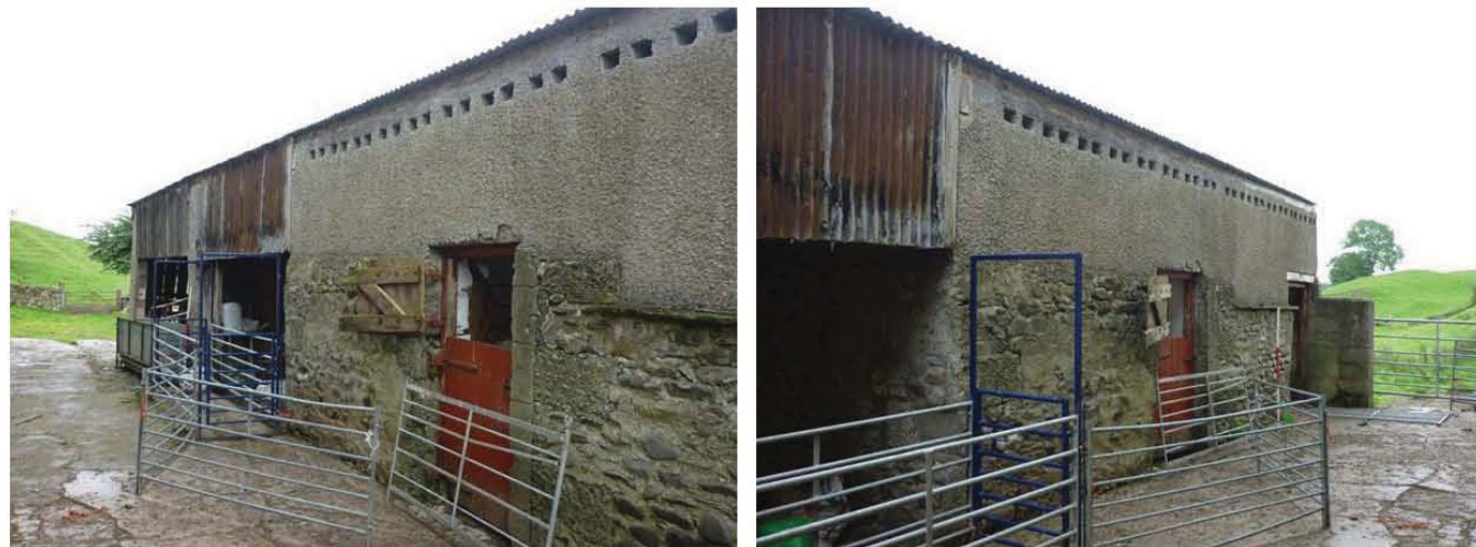
Plate 32 (left): North end of the west external elevation of the east outbuilding
