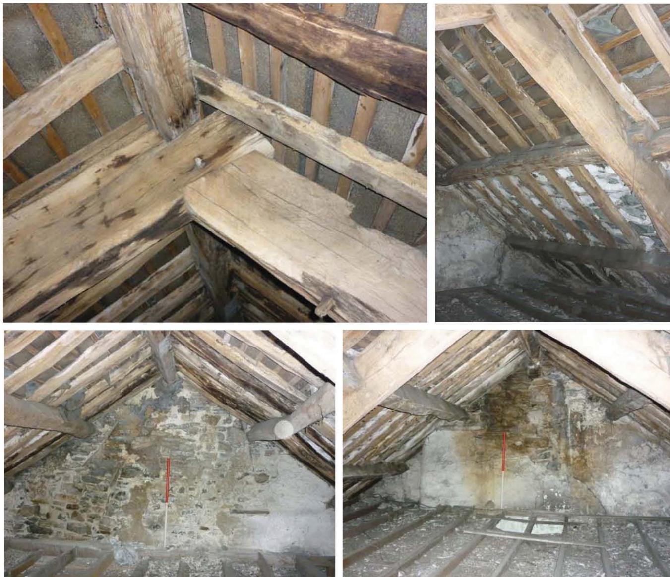
Plate 64 (top left): Detail of lap joint in the truss above first floor Rooms 4 to 7 of the farmhouse
