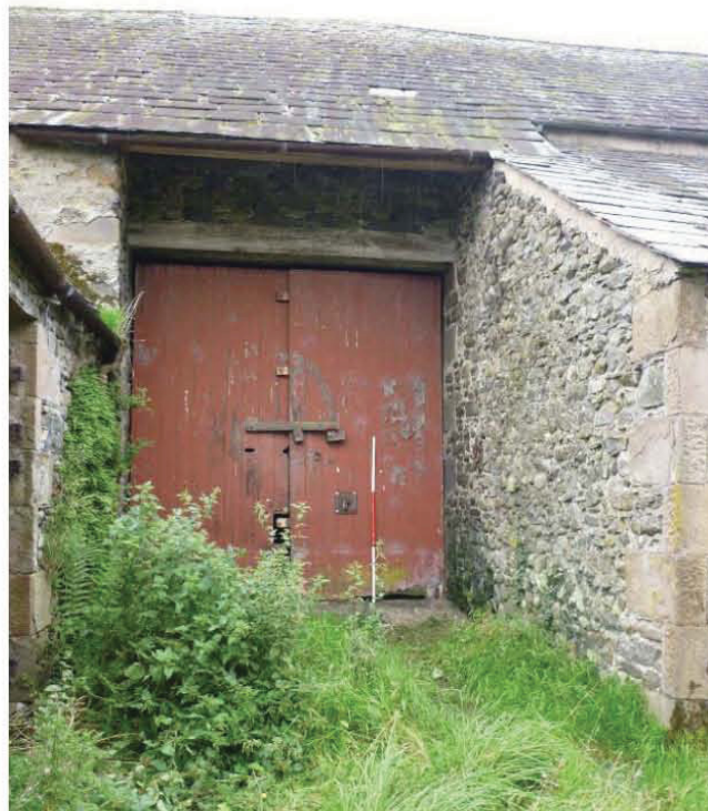
Plate 14 (top left): East end of the north external elevation of the barns
