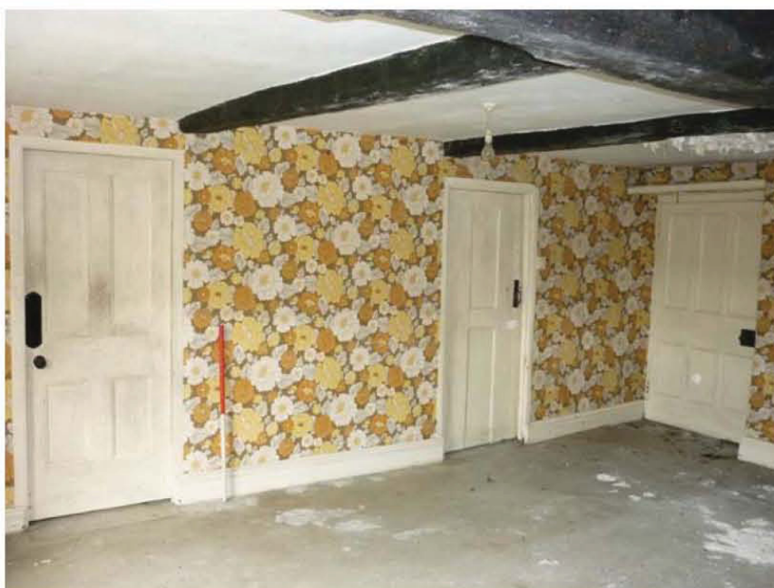
Plate 44 (top left): East elevation of ground floor Room 3 of the farmhouse, showing the bressummer beam
