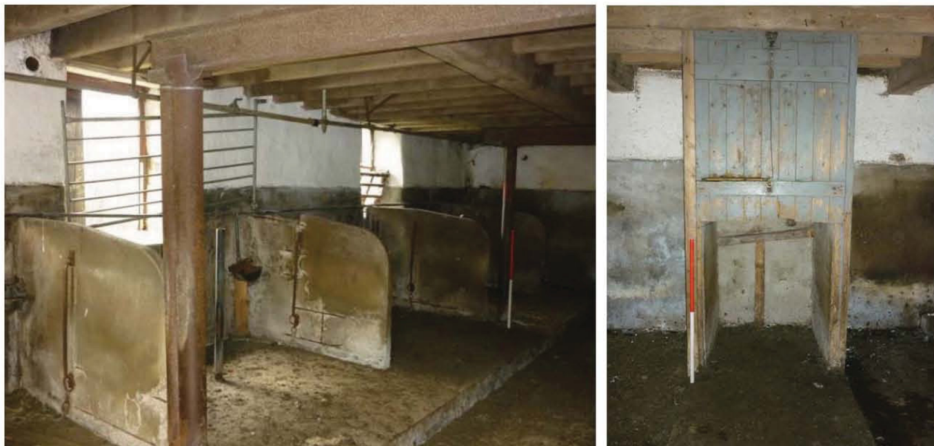
Plate 92 (left): Concrete stalls against the south wall of lower floor Room 4 of the barns
