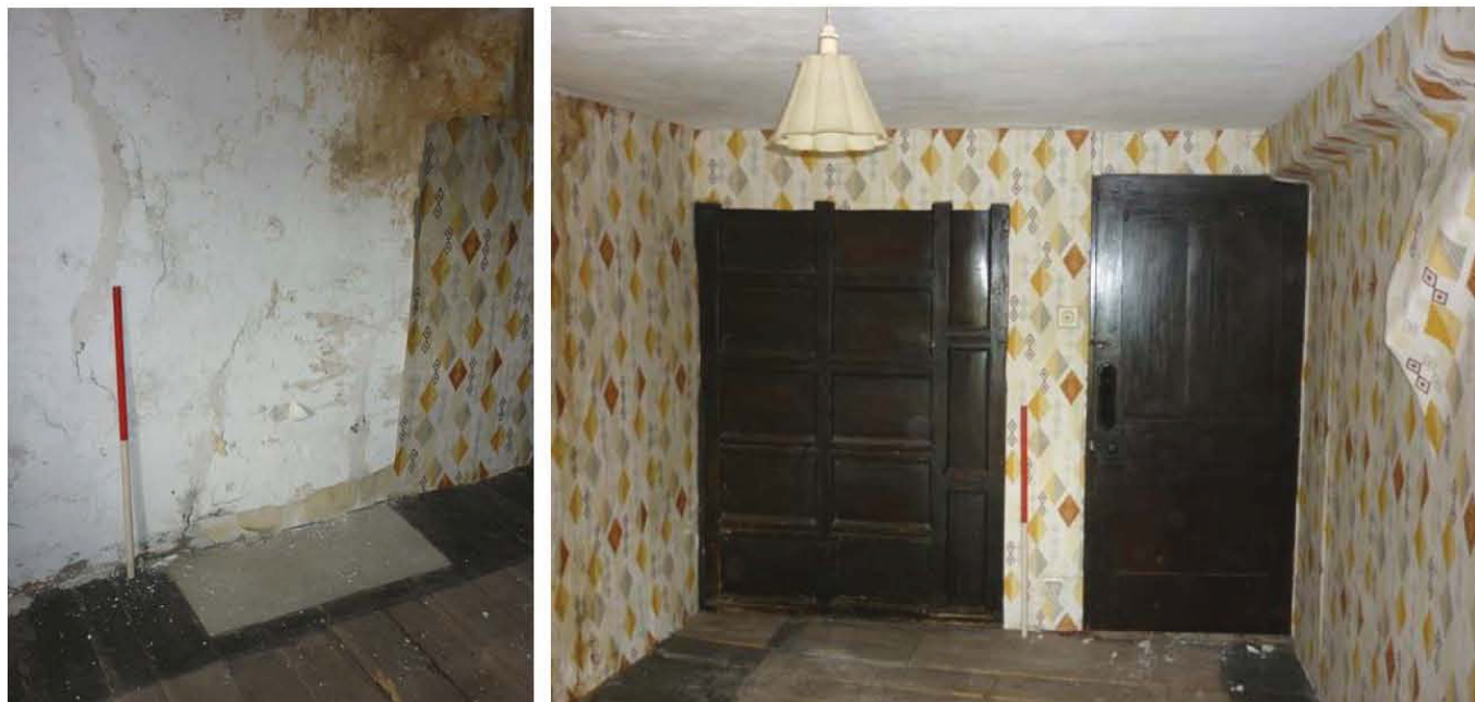
Plate 53 (left): Concrete hearth in the west elevation of first floor Room 3 of the farmhouse
