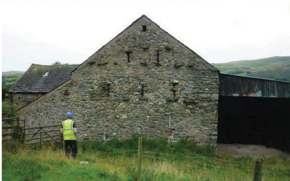
Plate 23 (top left): North end of the east external elevation of the barns
