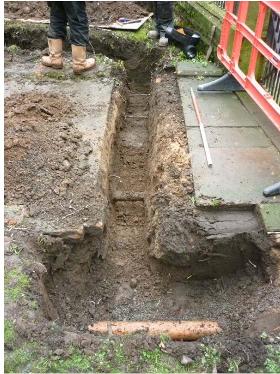
Plate 6: Excavation below the north end of the footpath, near to the boundary wall
