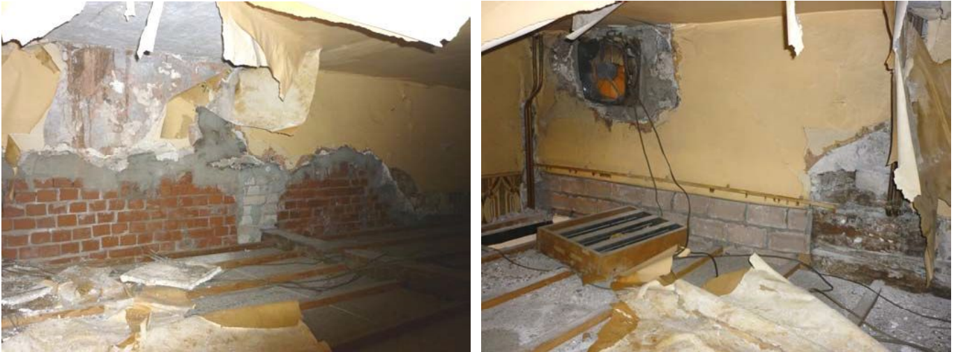
Plate 34 (left): Rebuilt section of the north elevation above the suspended ceiling in Room G7
