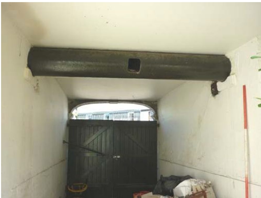
Plate 27: General view of Room G4, showing the gated entrance and pipe supported by corbels below the ceiling
