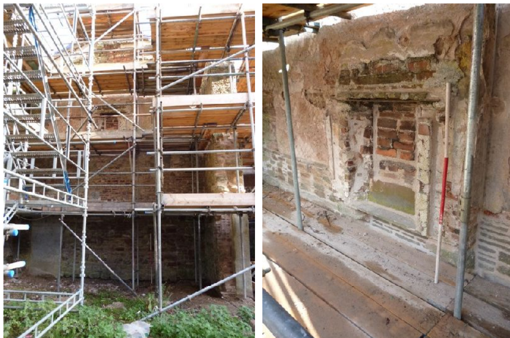
Plate 31 (left): West elevation of the projecting section at the north end of the west external elevation
