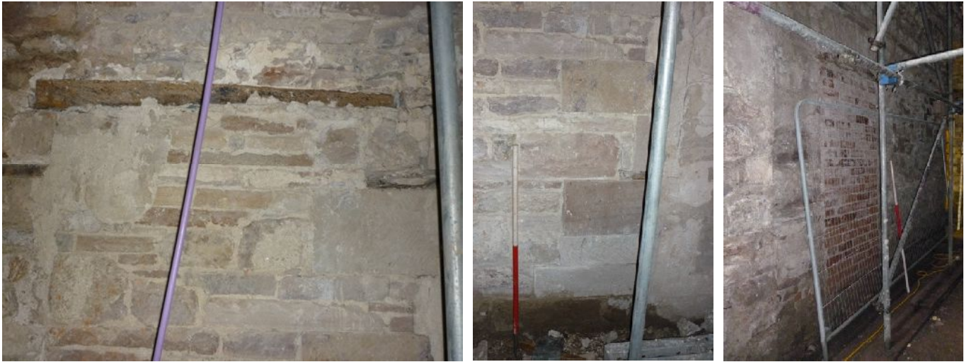
Plate 49 (left): Timber in the west elevation at the south end of Room 1 (photograph taken 25 th August 2011)
