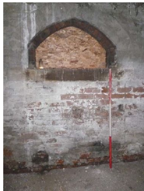
Plate 19 (right): Boarded up window on the north-west elevation
