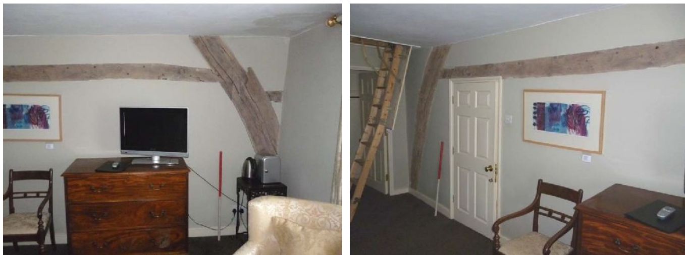
Plate 28 (left): End of cruck with spur and collar exposed at north end of west elevation, Room F4
