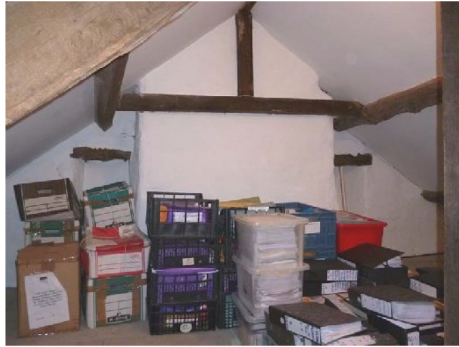
Plate 34: South end of southern section of roof space, showing chimney breast with flanking windows
