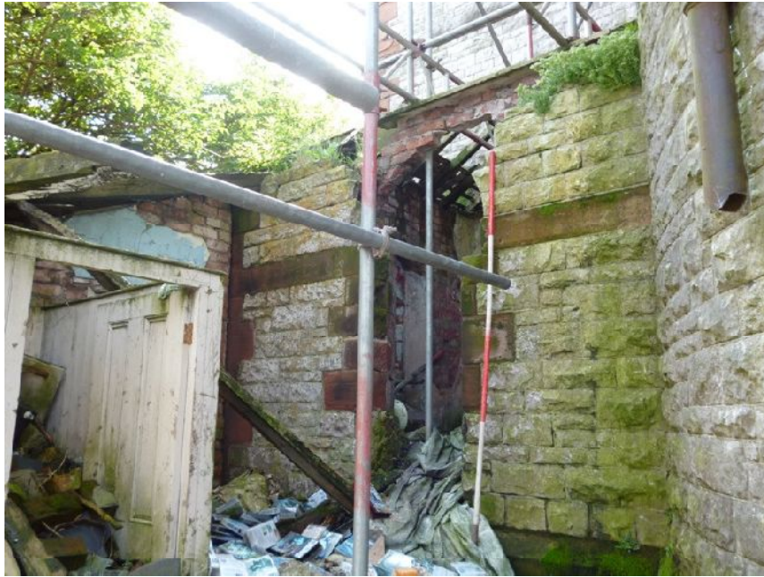
Plate 16 (left): Damaged window, on the south-east side of the north-east external elevation, latterly used as a doorway between G4 and G5
