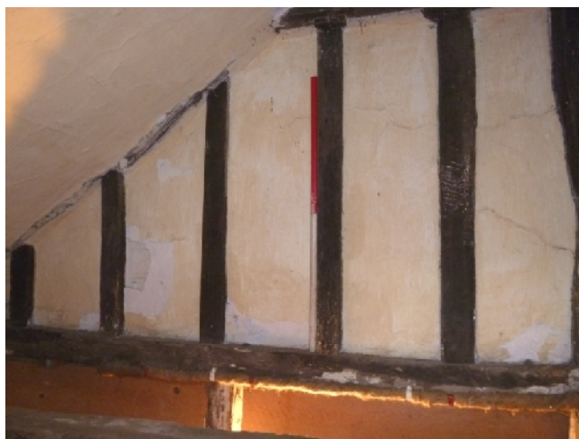
Plate 27: Stud wall above the door to the cellar, viewed from the stairs to Ground Floor Room G8
