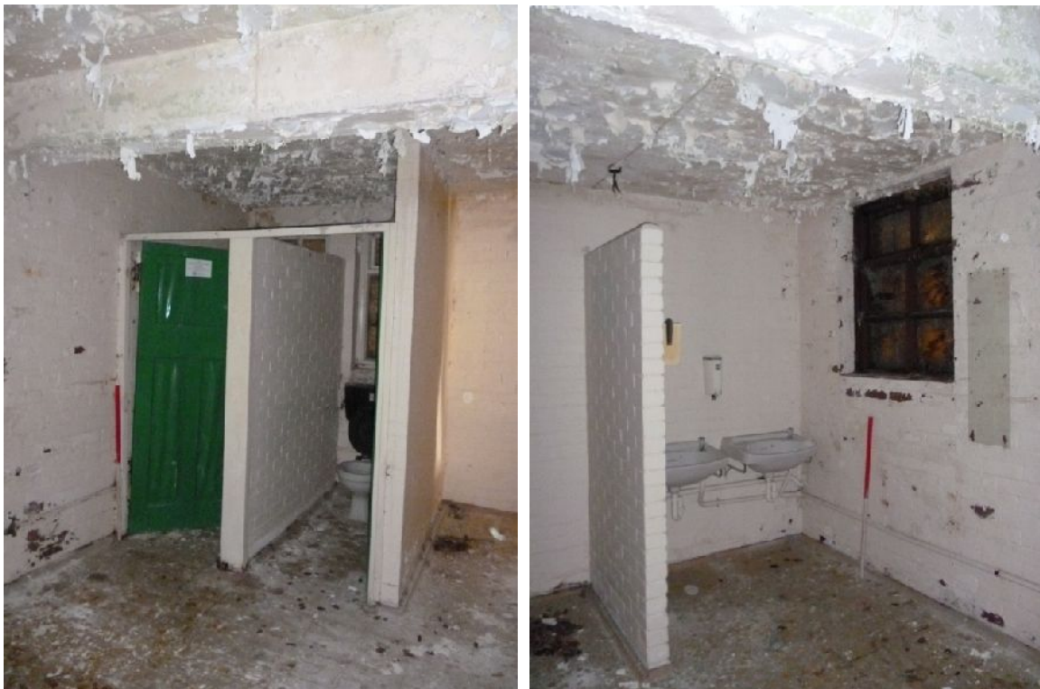
Plate 88 (left): Toilet cubicles to the east side of North Building, Ground Floor Room 3
