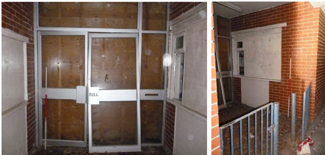
Plate 179 (left): Double door in the west elevation return of West Building, Ground Floor Room 1
