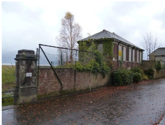
Plate 28: Oblique view of the upper floor of the north elevation and west elevation of the north building
