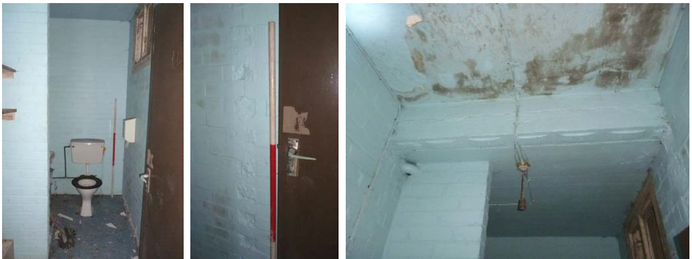
Plate 186 (left): Toilet against the north elevation of West Building, Ground Floor Room 3
