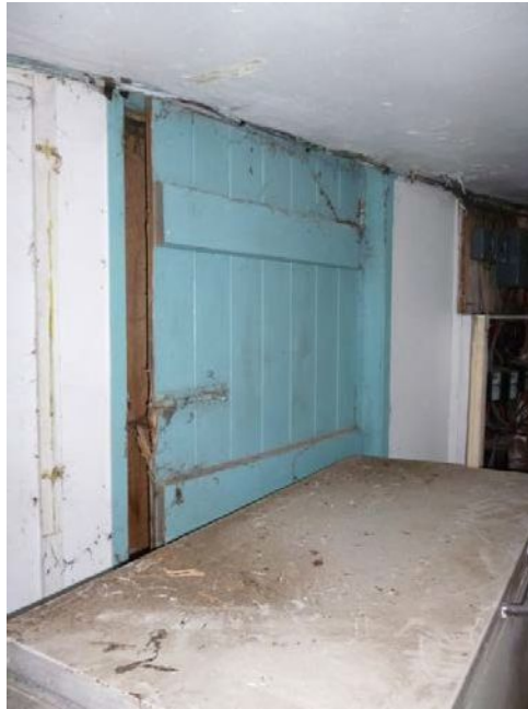
Plate 151: Plank and batten door in the west elevation of South Building, Ground Floor Room 9
