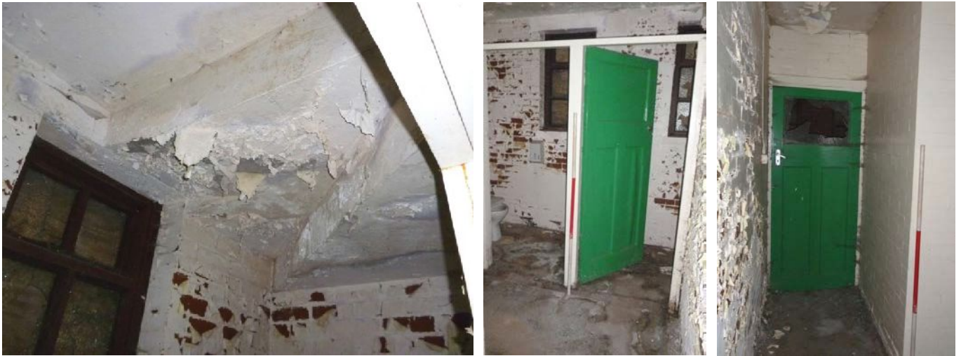
Plate 183 (left): Underside of the steps visible in West Building, Ground Floor Room 2
