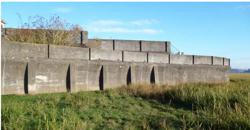
Plate 77: The south side of the outer retaining wall with concrete block wall on top
