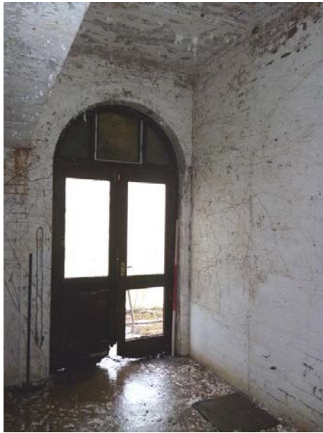
Plate 112: Doorway on the north side of the west elevation, northern half of the ground floor room, east building
