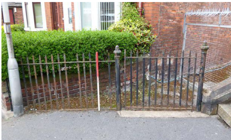
Plate 21: Cast iron fence at the north-west end of the south-west external elevation
