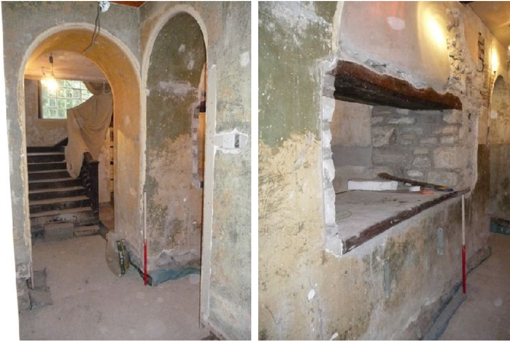
Plate 27 (left): Arches at the end of the east/west section of ground floor Room 2
