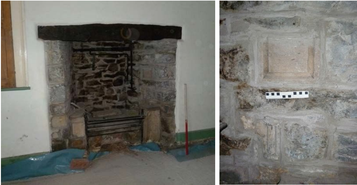
Plate 43 (left): Fireplace on the north elevation of Room 6 on the ground floor
