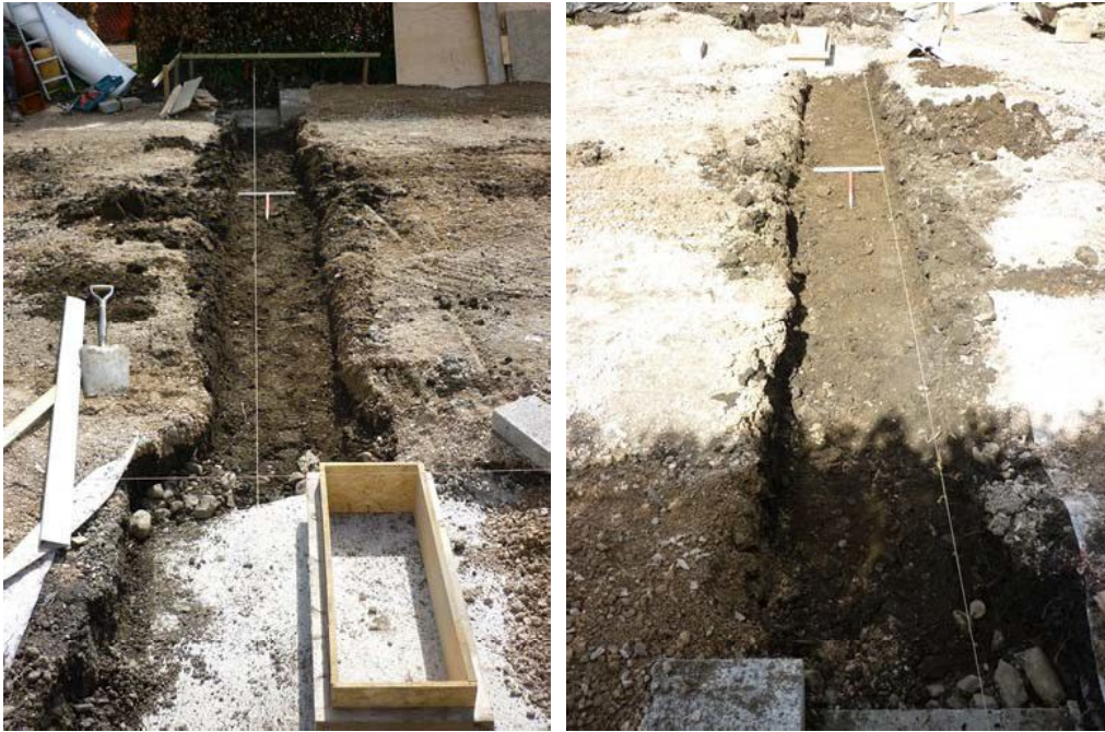
Plate 14 (left): Area excavated between the north- and south-east pits, viewed from the north
