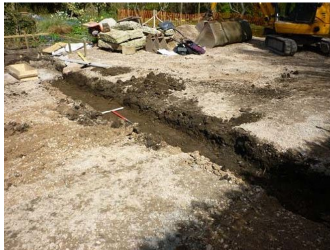
Plate 16: Area excavated between the north- and south-east pits, viewed from the south-west
