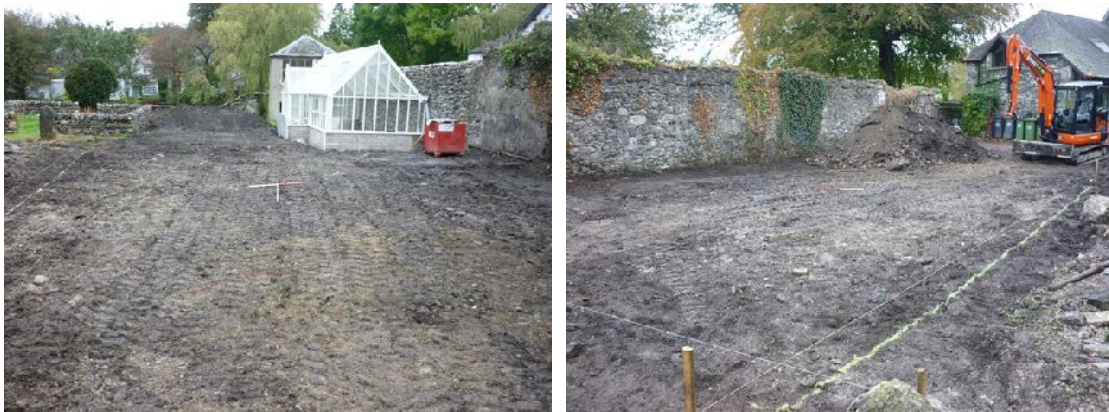
Plate 18 (left): Area of the new garage/workshop prior to excavation, viewed from east
