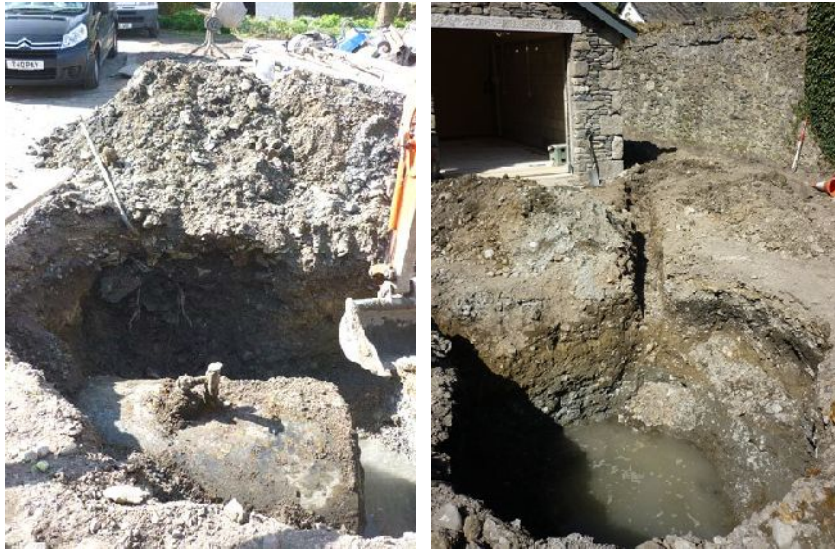
Plate 47 (left): Stony deposit (126) visible in section (to the left hand side) near the disused fuel tank
