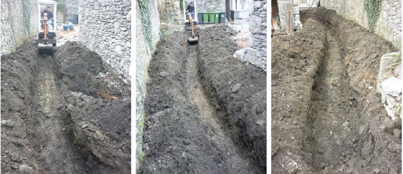
Plate 42 (left): Excavation of service trench to the north of the new garage
