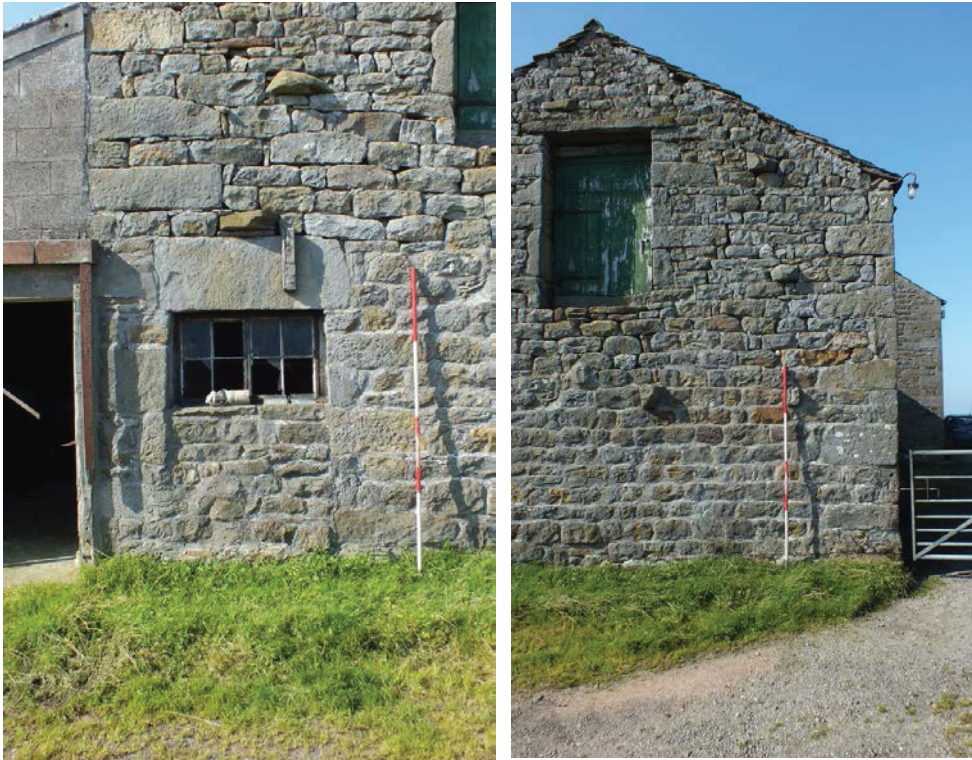
Plate 6 (left): Blocked doorway to the barn on the ground floor of the north-east external elevation
