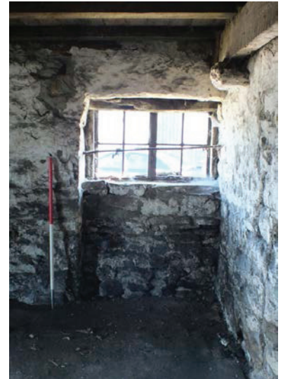
Plate 15 (right): Blocked feature at the south-east end of the north-east elevation (G1)
