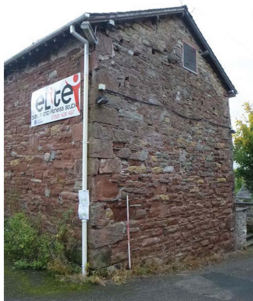
Plate 20: The west external elevation of the main section, viewed from the north-west
