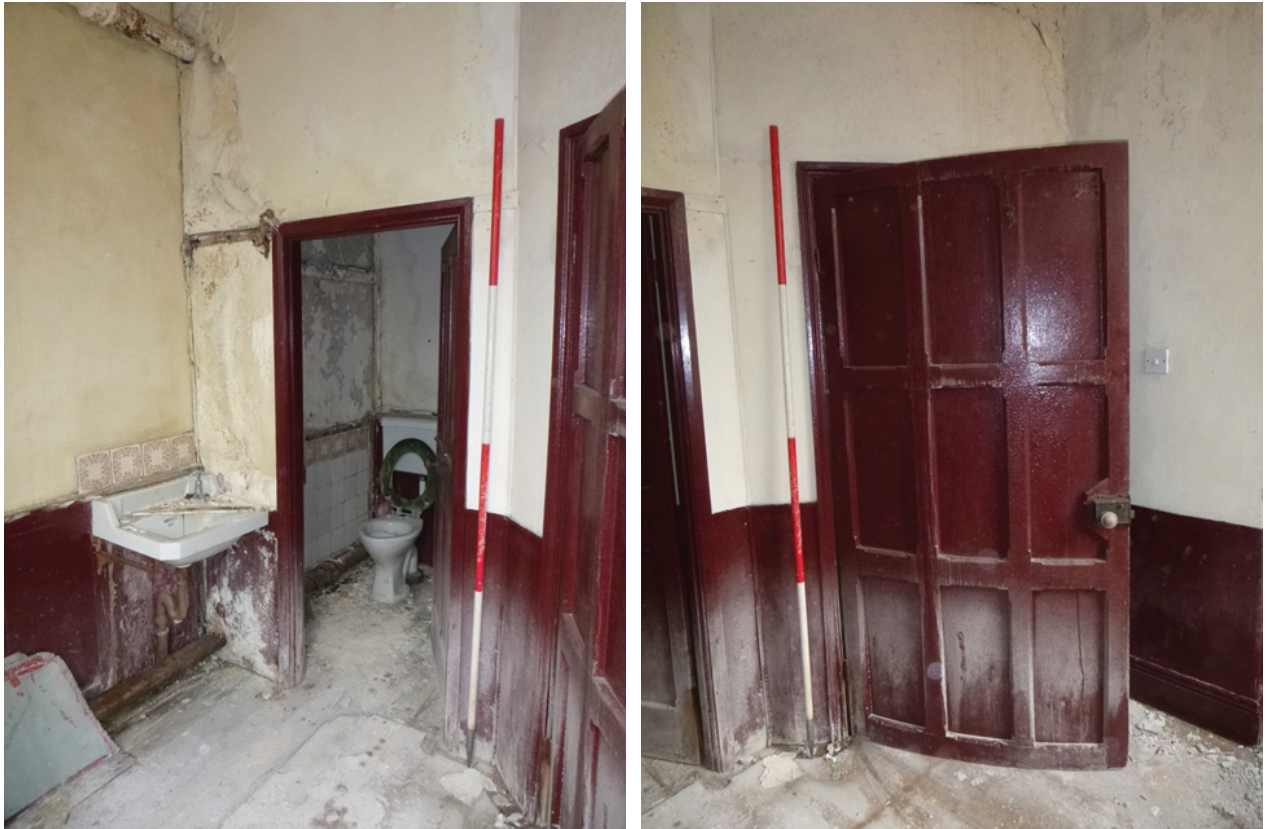
Plate 79 (left): Toilet and sink in the north-west corner of ground floor Room 4, viewed from the south-east Plate 80 (right): Curved door in the east side of the north elevation, ground floor Room 4, viewed from the south-west
