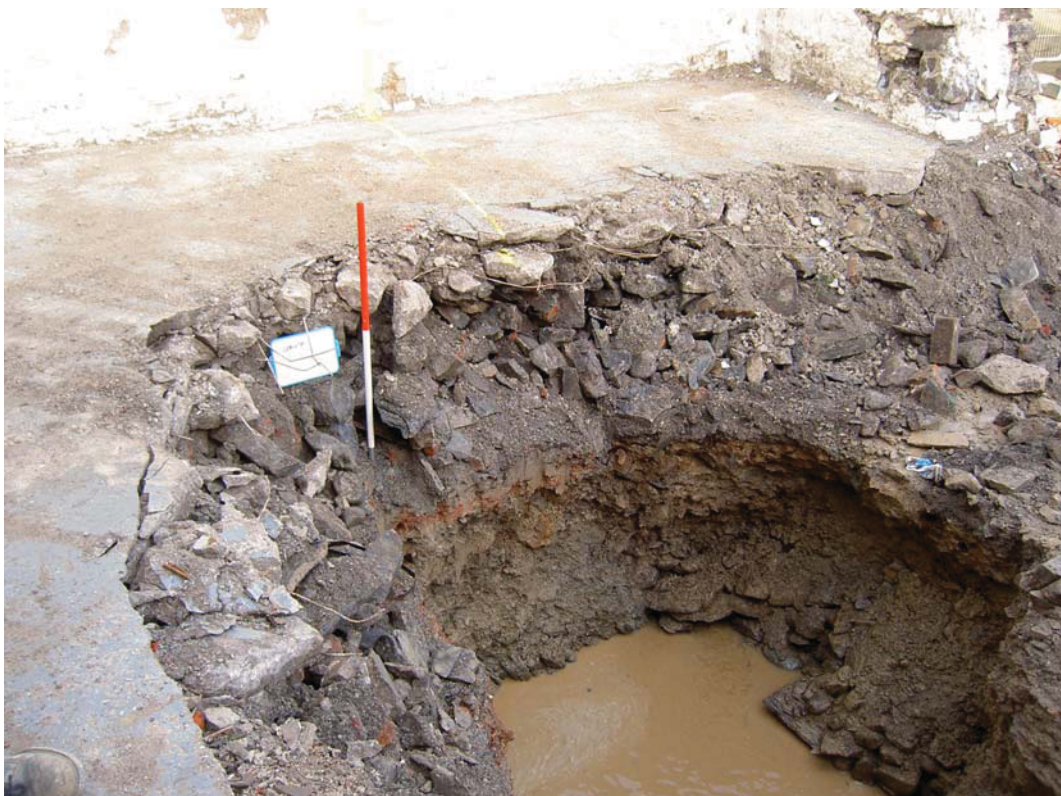
Plate 11: Trench 1, following culvert damage
