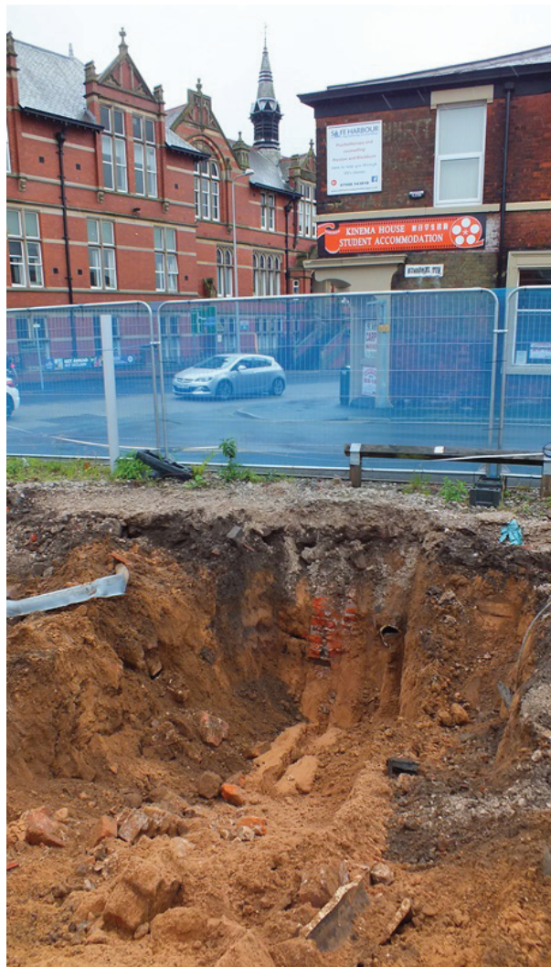
Plate 10: Wall, ceramic drain and other services adjacent to Edward Street, viewed from the east
