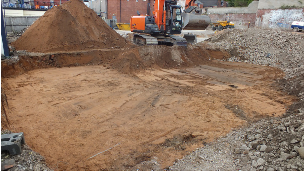
Plate 15: Excavation at the site entrance from Edward Street, viewed from the west
