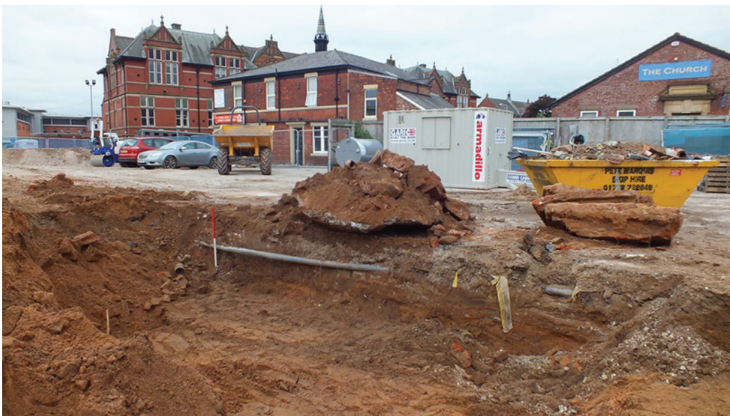
Plate 14: Wall and service pipe at the edge of the car park off Edward Street, viewed from the east
