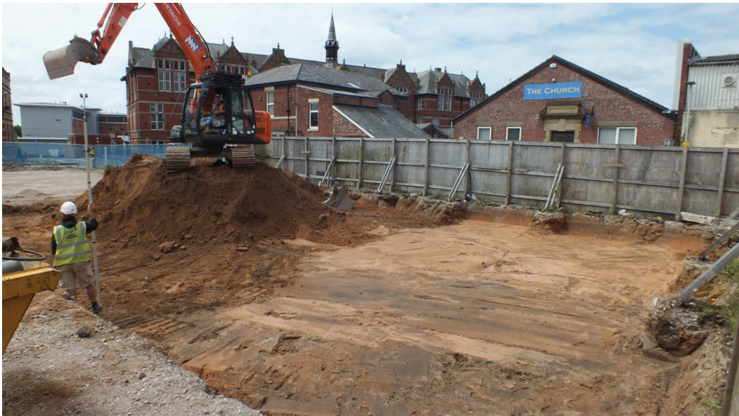
Plate 16: Excavation at the north end of Edward Street, viewed from the south-east
