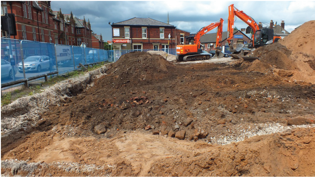
Plate 9: Removal of rubble and hardcore along Corporation Street, viewed from the south-east
