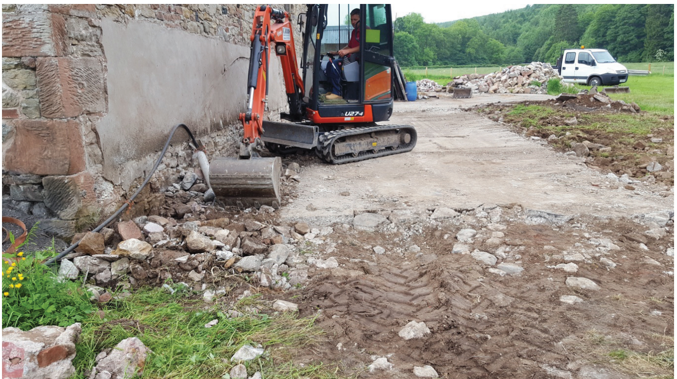
Plate 9: The removal of the concrete foundations for the steel-framed lean-to on the western side of the barn (photograph: J. Beaty)
