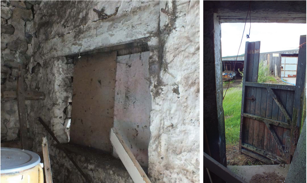
Plate 31 (left): Window at the west end of the north elevation in G4
