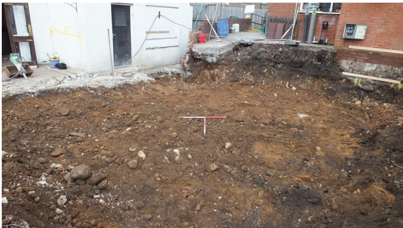
Plate 15: East side of the area stripped to the south side of the Boot and Shoe Hotel
