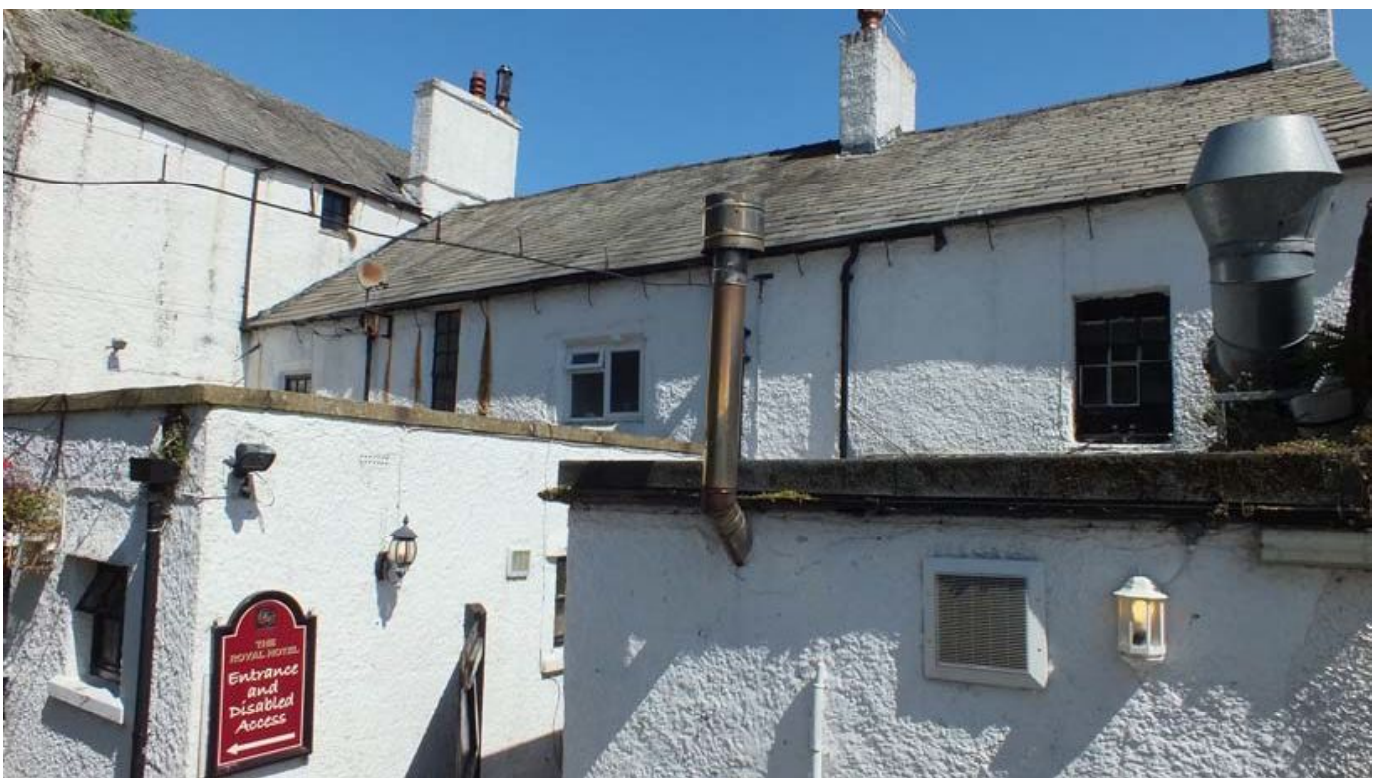
Plate 21: The west external elevation of the main building of the Royal Hotel
