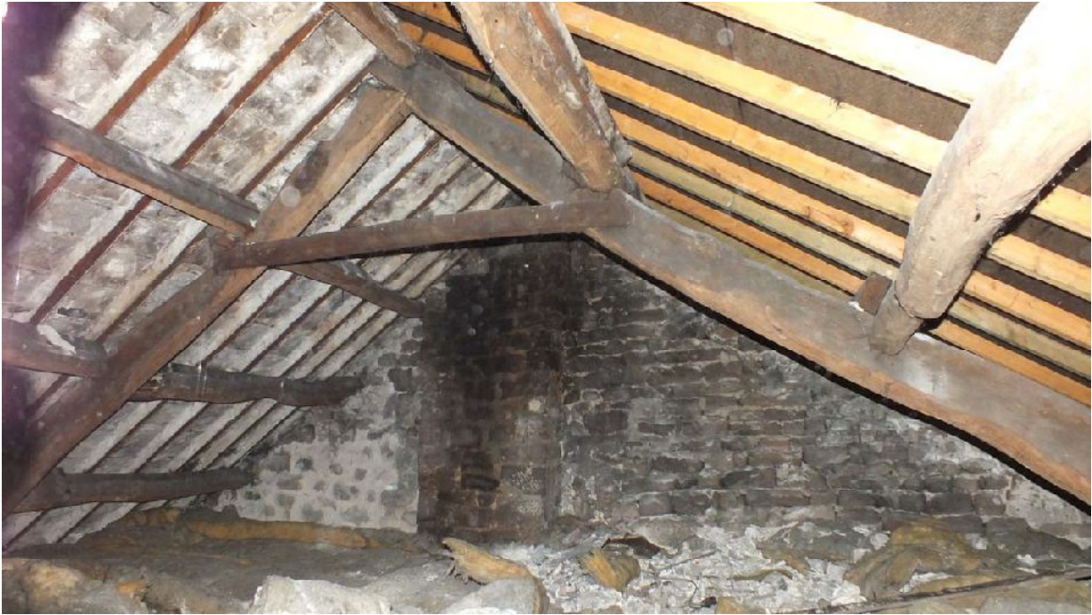
Plate 108: Truss and chimney breast in the south part of the roof space
