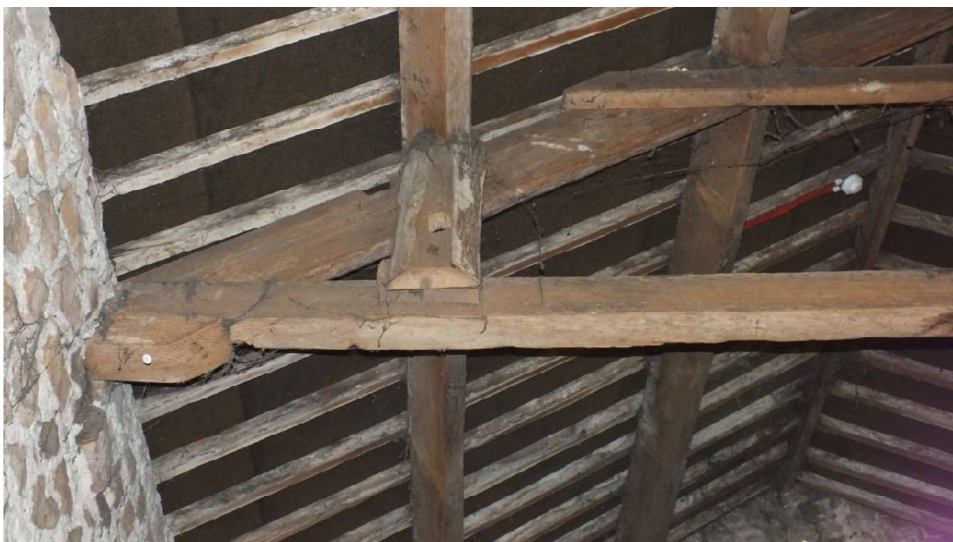
Plate 75: Timber corbel below the east end of the truss on the south side of F3
