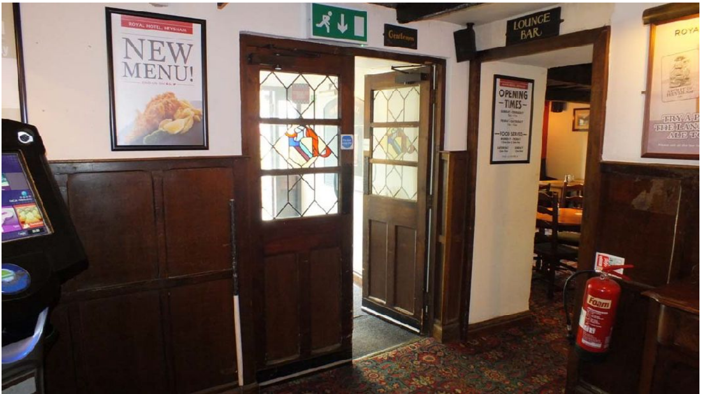
Plate 44: Doorways to the porch and G4 at the north end of G5
