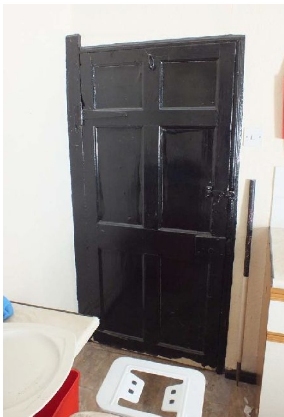
Plate 84: Panel door in F5
