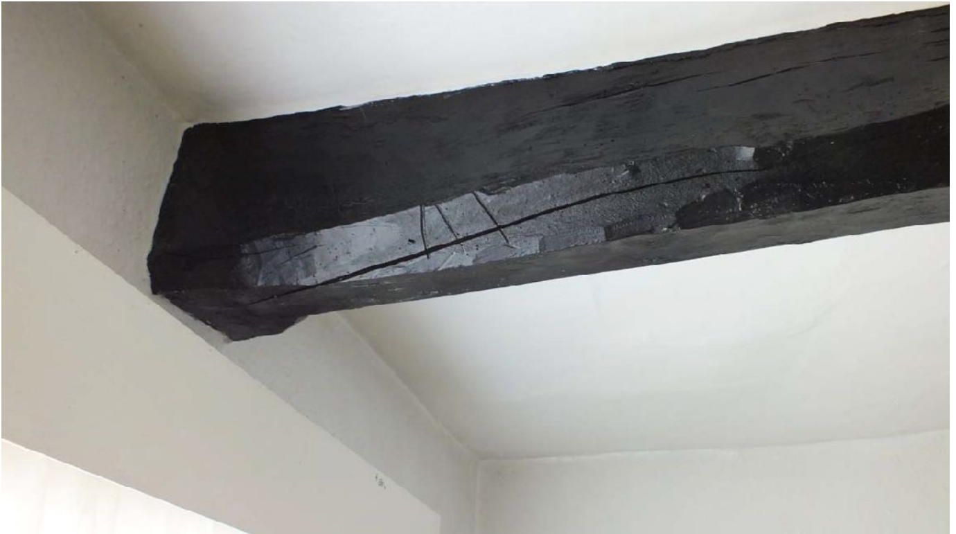
Plate 88: Detail of the Baltic marks at the east end of the central beam in F7
