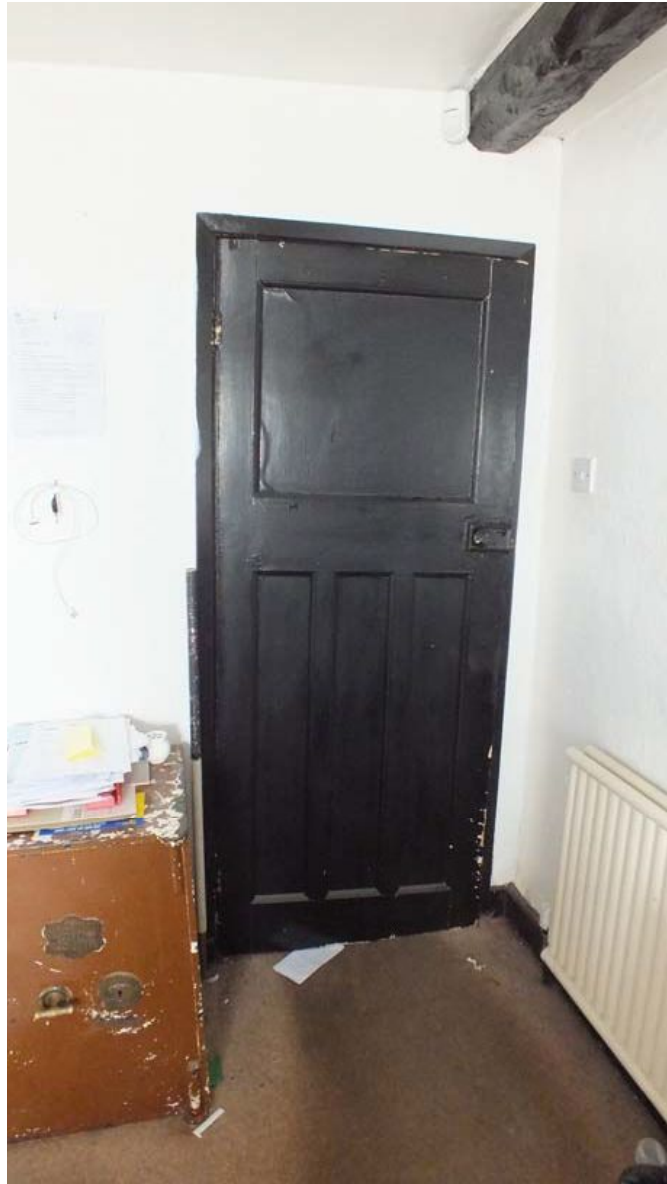
Plate 89: Panel door in F7
