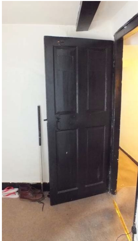
Plate 97: Panel door in F10
