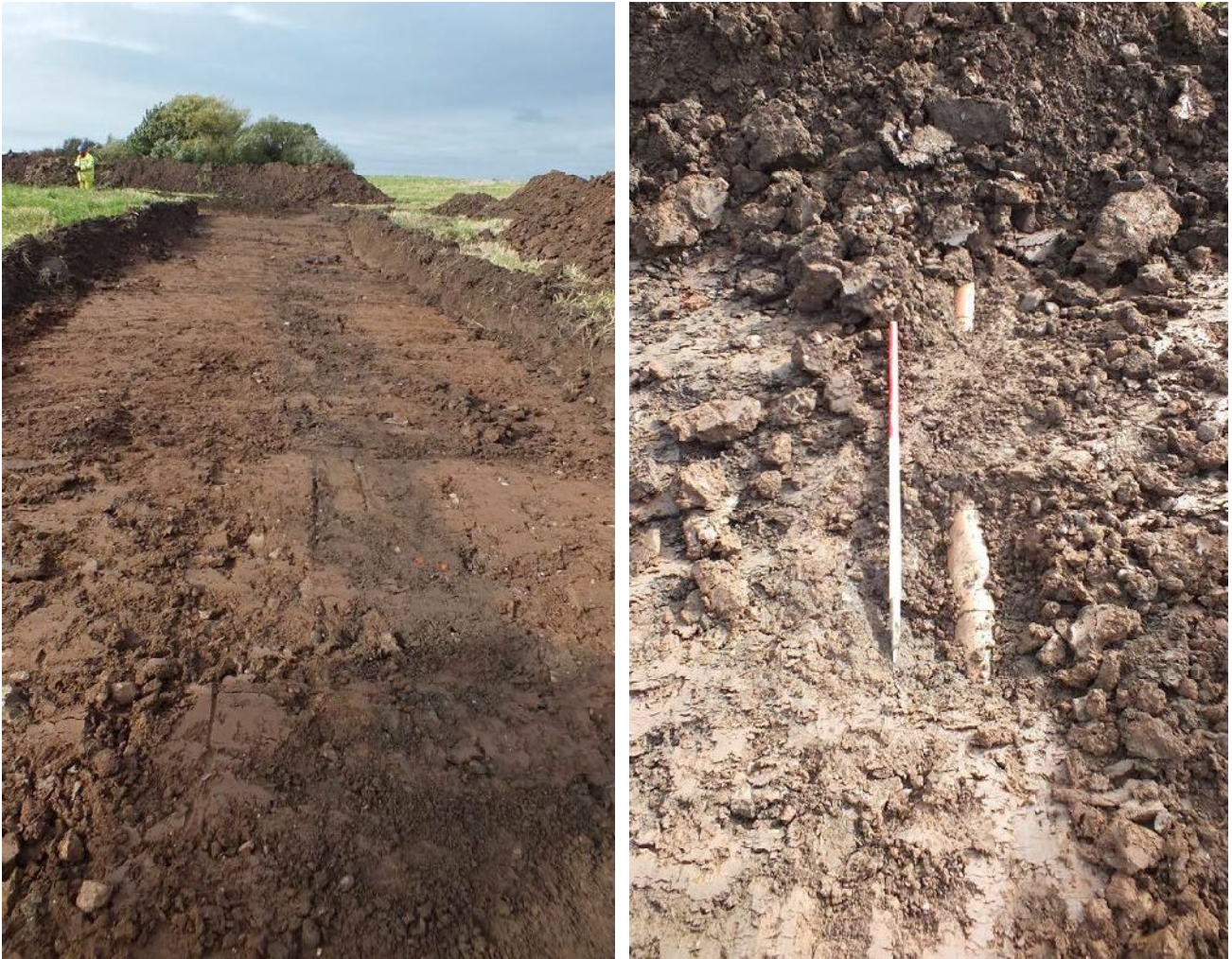
Plate 15 (left): Cut of pipe trench running through 107 and 108, viewed from the south-east
