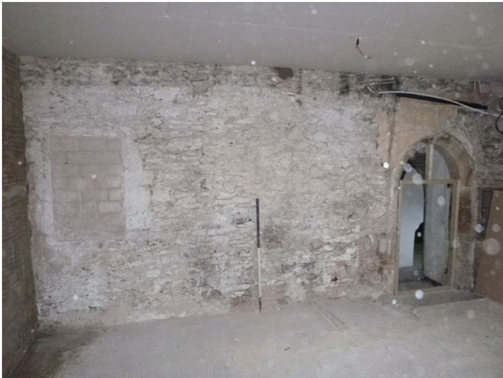
Plate 30: View of the whole of the south wall of the kitchen stripped of plaster, from the north-west
