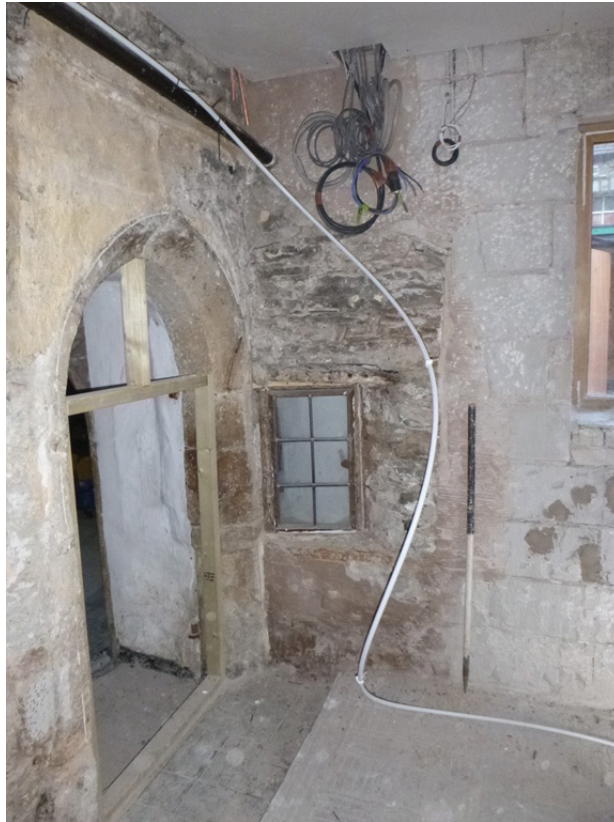
Plate 33: The west corner of the kitchen showing the junction of the stub wall to the original north-west wall and extension of 1970, viewed from the east
