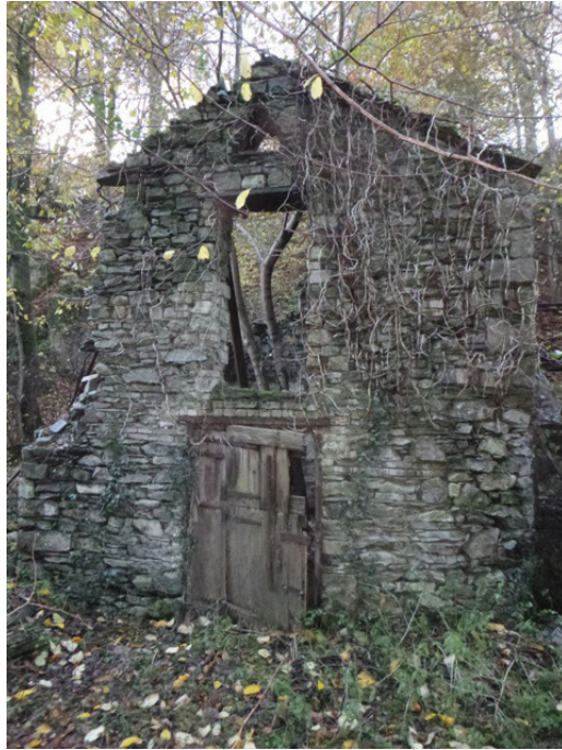
Plate 16: The two-storey south-east end of the south block, viewed from the east
