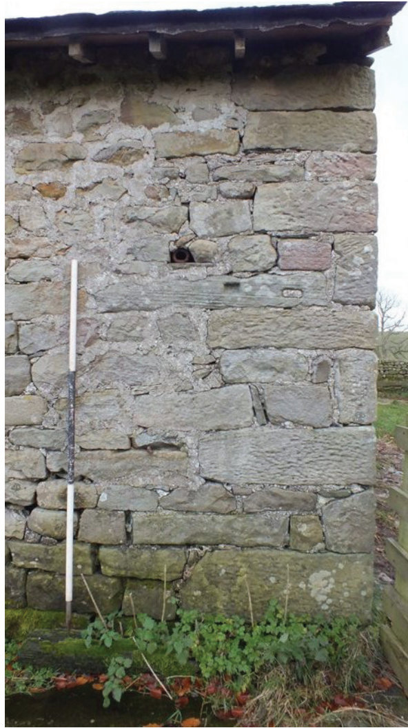
Plate 18: Re-used stone at the south end of the west external elevation, viewed from the west
