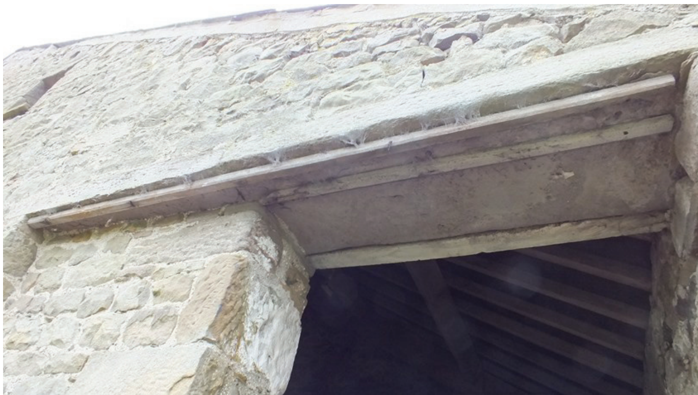
Plate 13: The lintel of the west doorway in the north external elevation, viewed from the north-west
