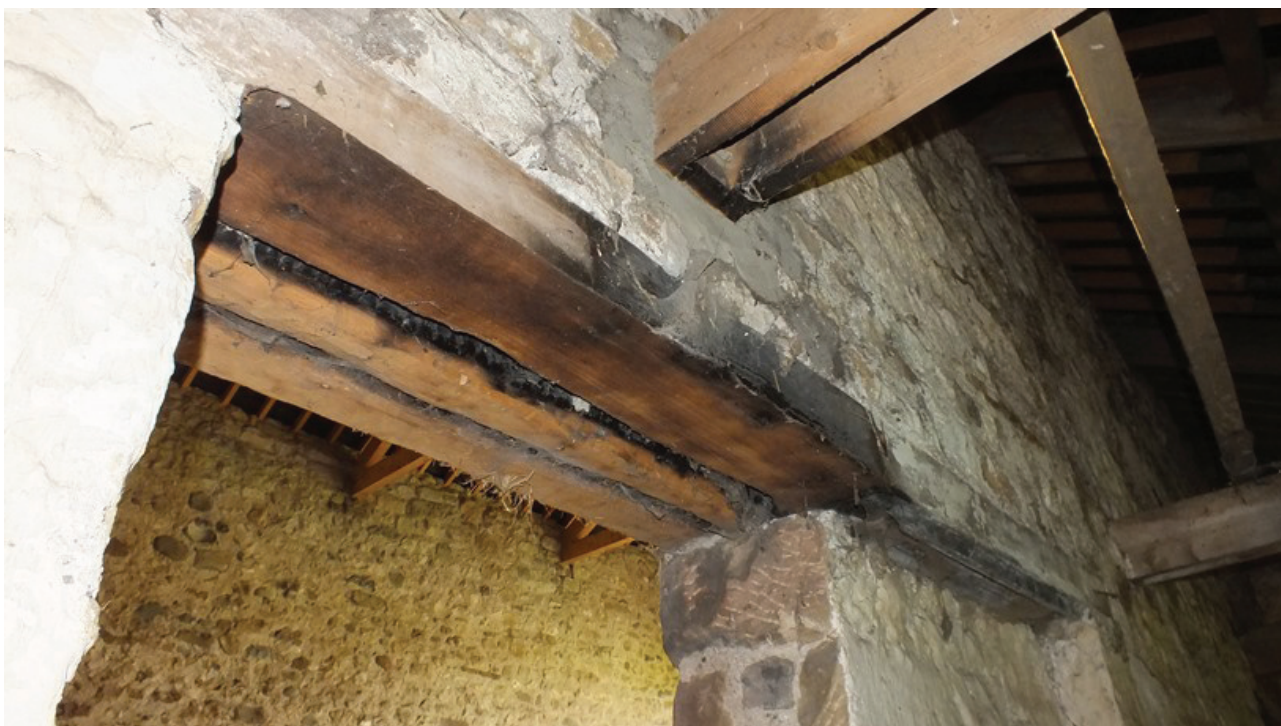
Plate 24: Detail of the lintel of the doorway on the south side of the west internal elevation showing the scorching, viewed from the south-east
