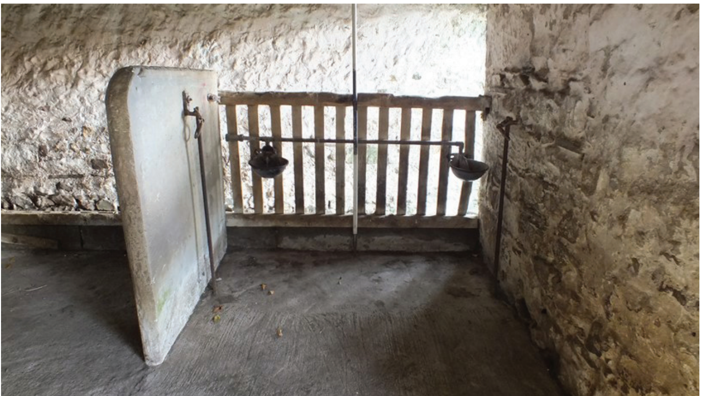
Plate 41: Detail of the intact stall at the south end of Room G4, viewed from the west
