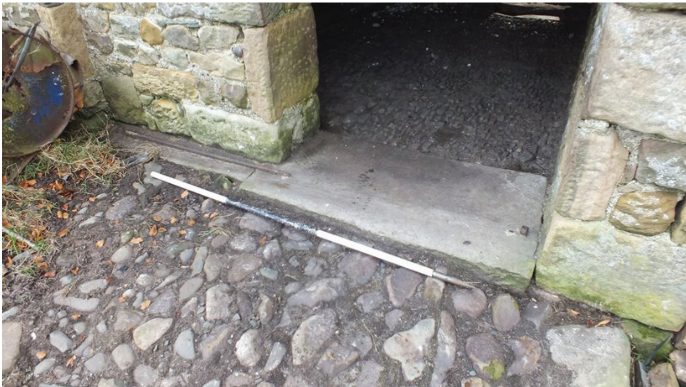
Plate 12: The threshold of the west doorway in the north external elevation, viewed from the north-west
