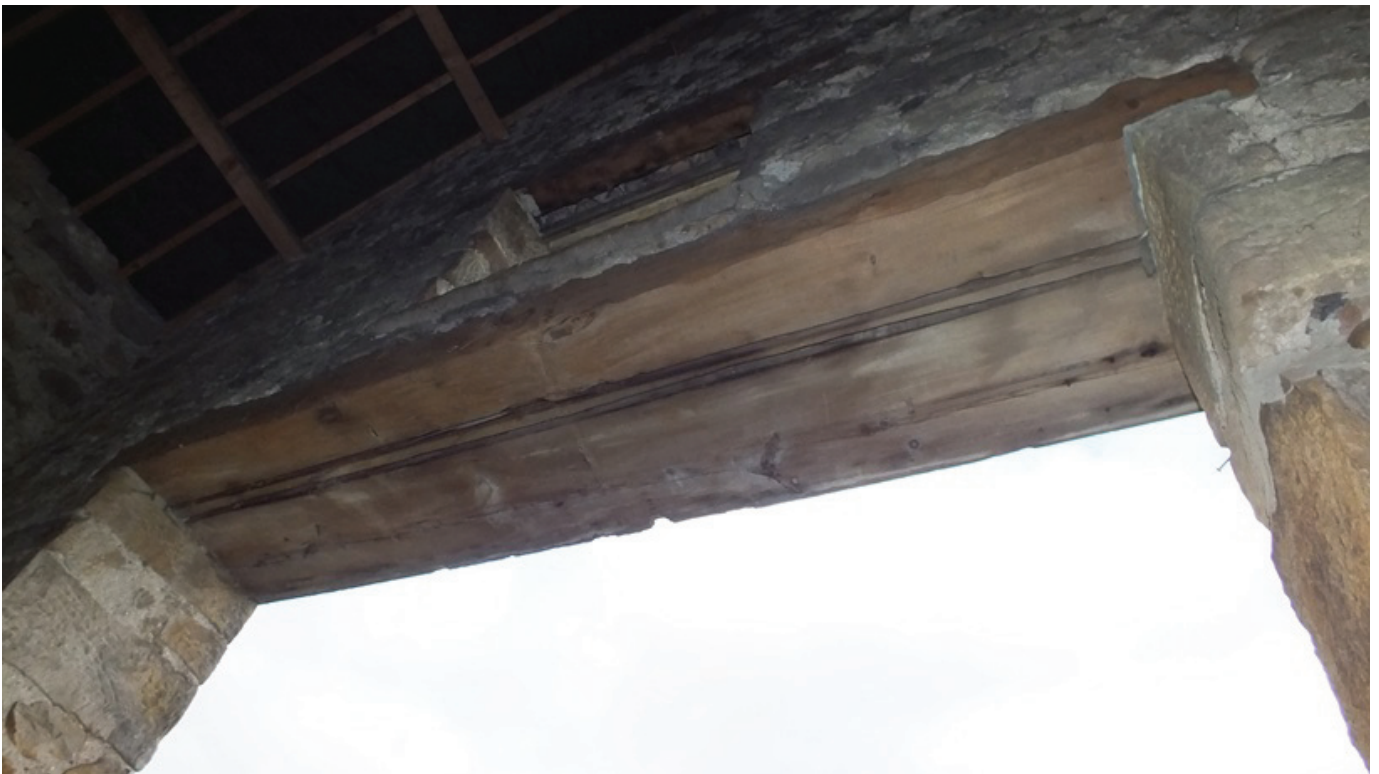
Plate 29: Detail of the lintel over the wagon doorway in Room G2 showing the grooves, viewed from the south-east
