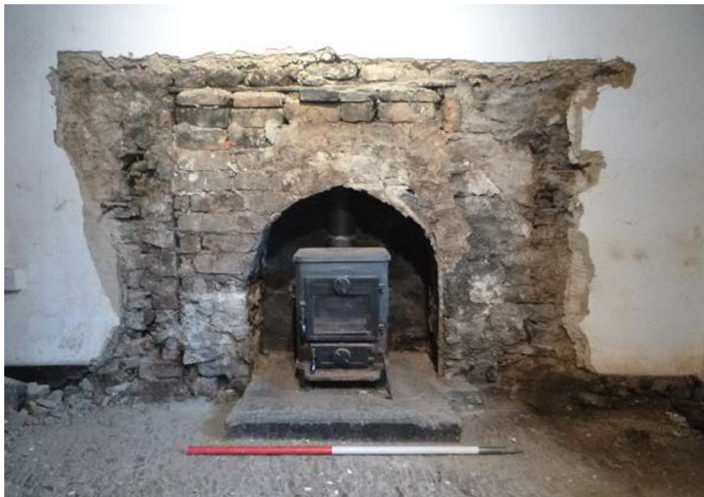
Plate 40: Fireplace in G4 after the timber and slate surround had been removed
