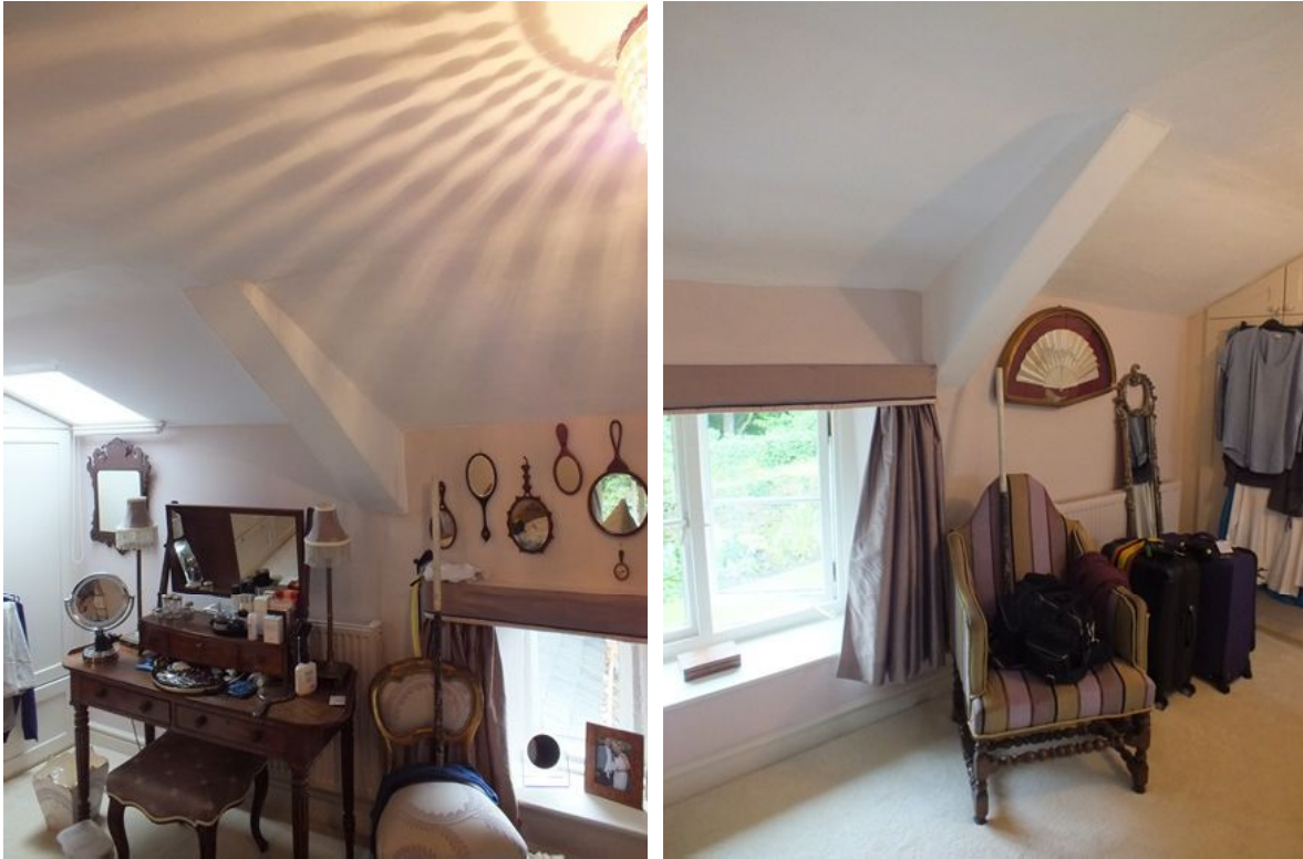
Plate 10 (left): The boxed end of the truss on the north-west side of the first floor, viewed from the east
