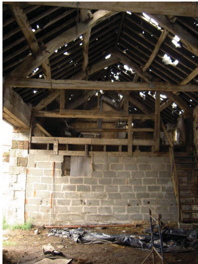
Plate 16: Inserted floor on top of blocking and re-used cruck blades in roof trusses of Building 2, looking north-west
