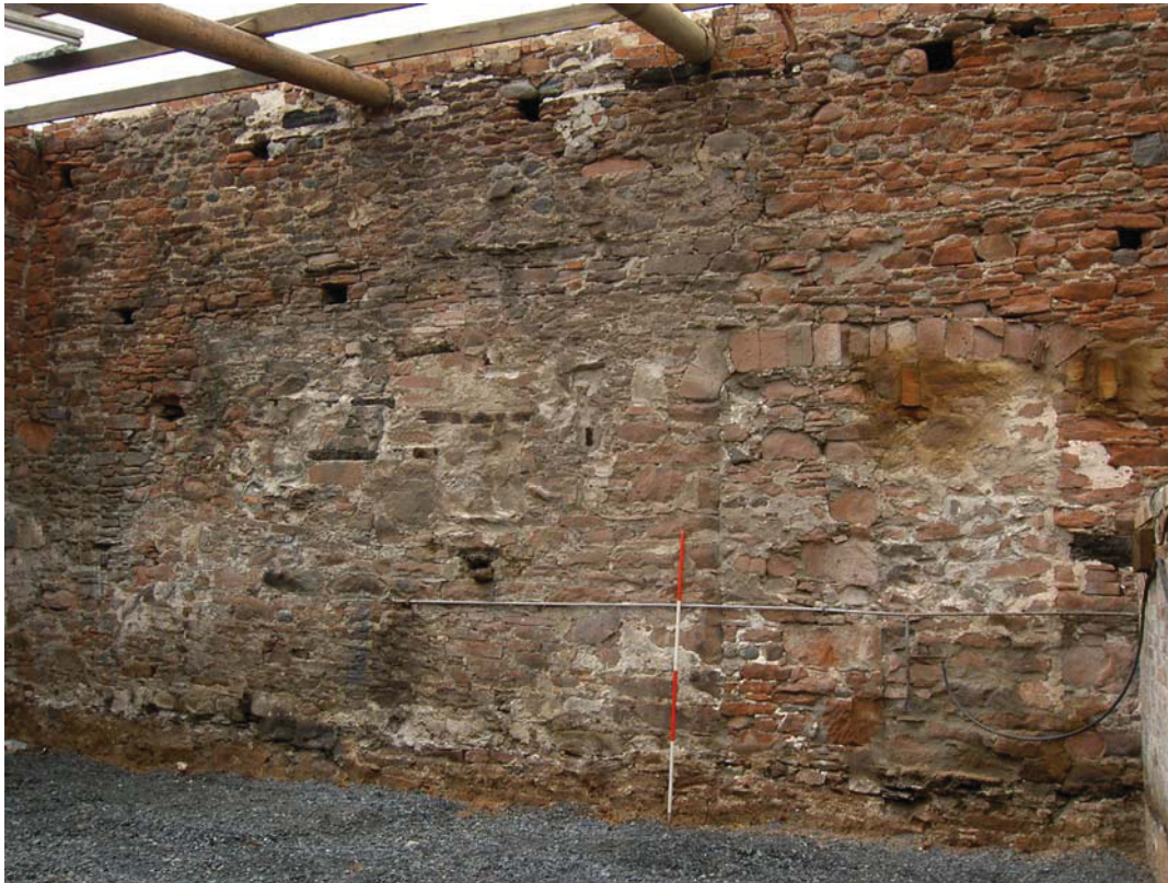
Plate 17: Interior of Building 4 showing original wall height and blocked double door and window, looking west
