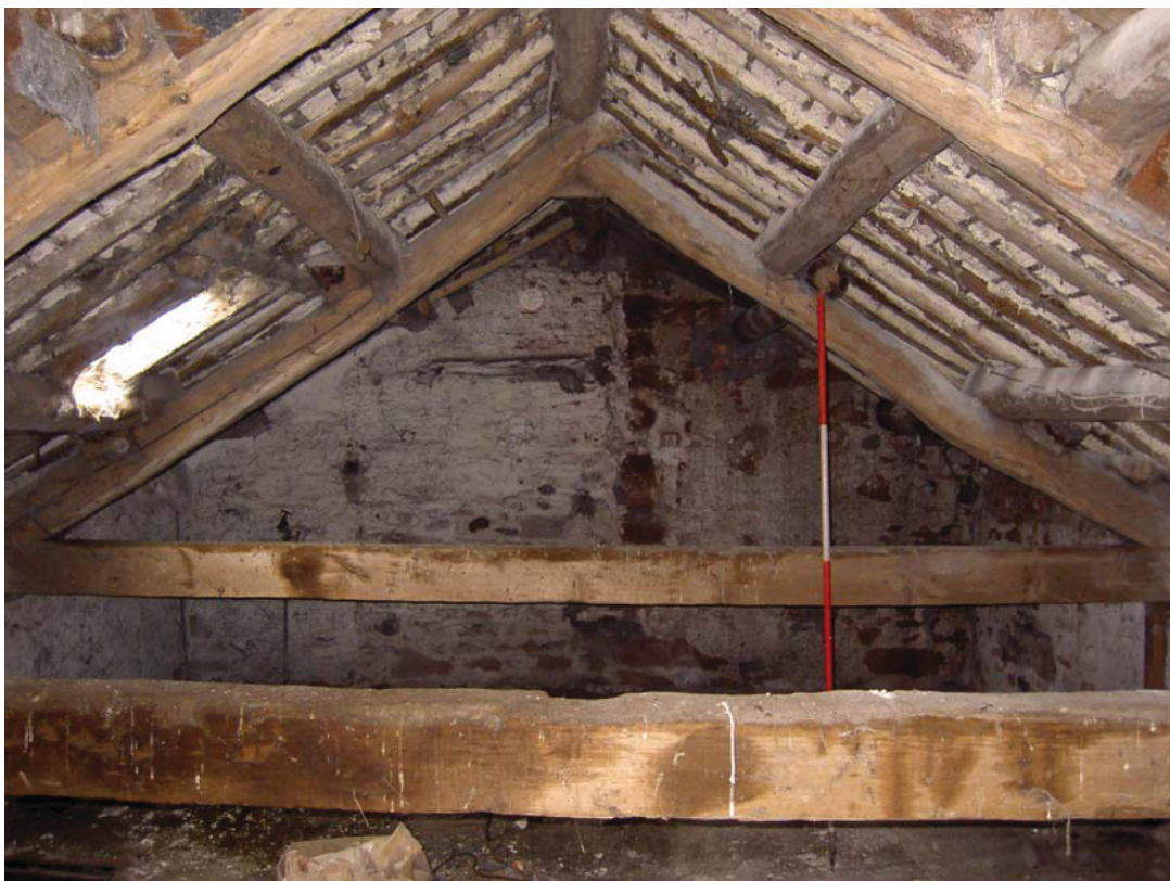
Plate 18: Detail of Building 5 roof structure and blocked window in west-north-west gable end of farmhouse
