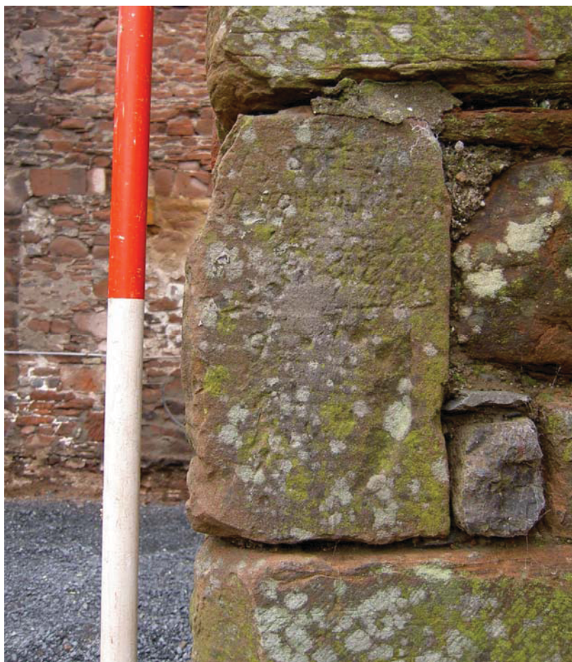
Plate 20: Graffiti on door quoin on the east-south-east elevation of Building 4
