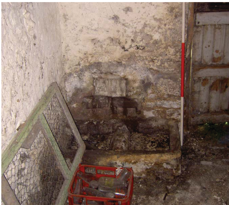
Plate 22: Blocked swill chute in north half of Building 1, from west
