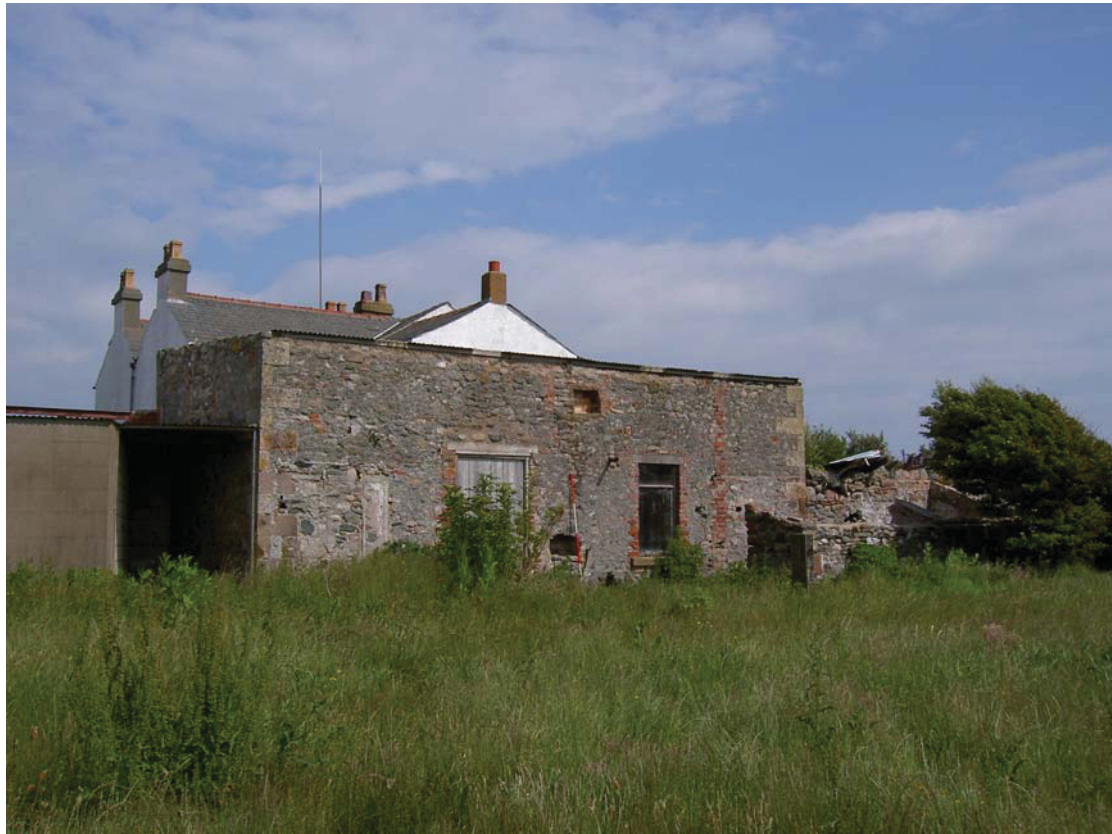
Plate 59: Derelict barn and outsheds to west of inn
