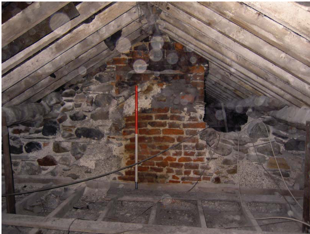
Plate 58: West end of roof space above first floor Rooms 8-10 showing original line of gable and brick flues
