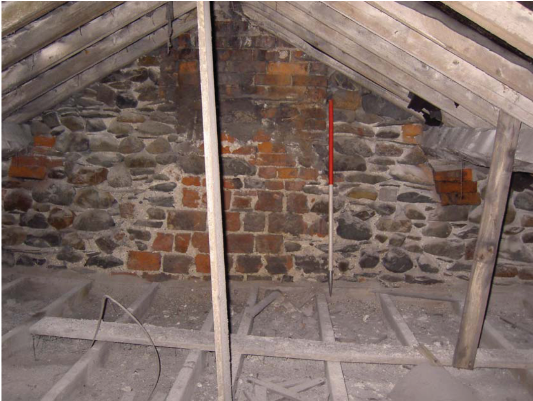
Plate 57: East end of roof space above first floor Rooms 8-10 showing original line of gable and brick flues
