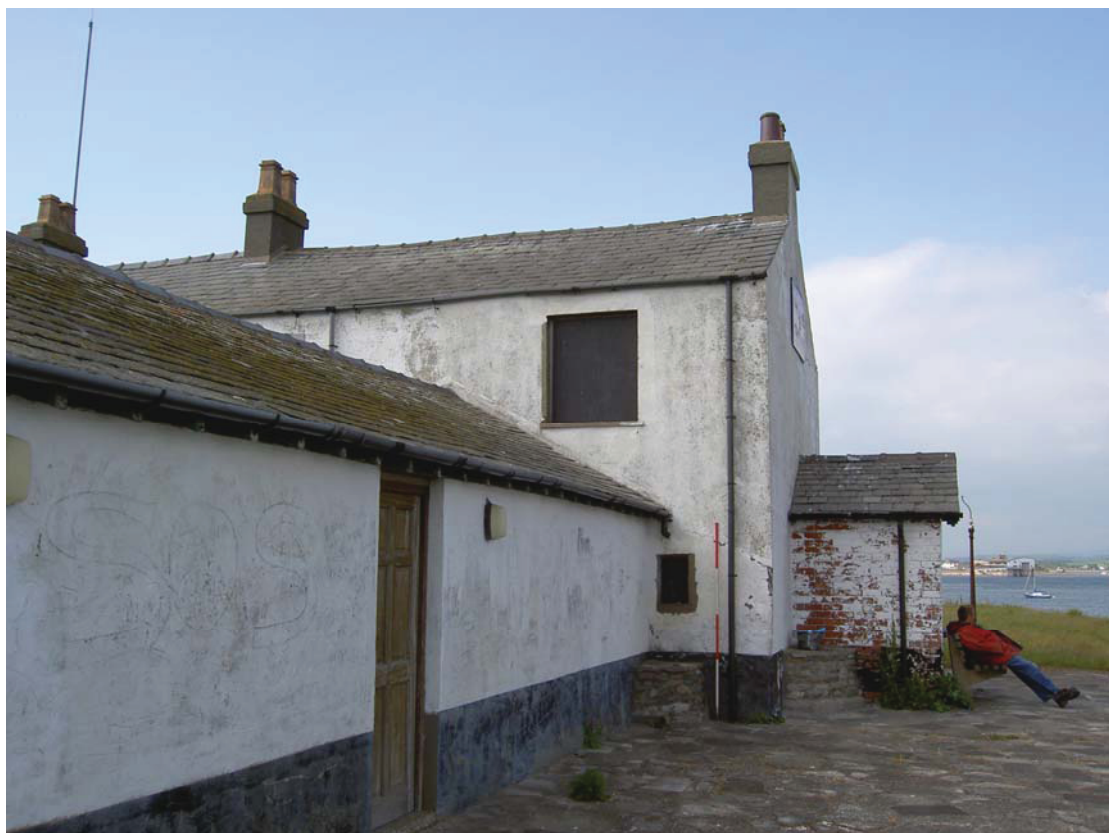
Plate 34: The east end of the south external elevation showing the repointed window surround above the pool room and the porch attached to the east end
