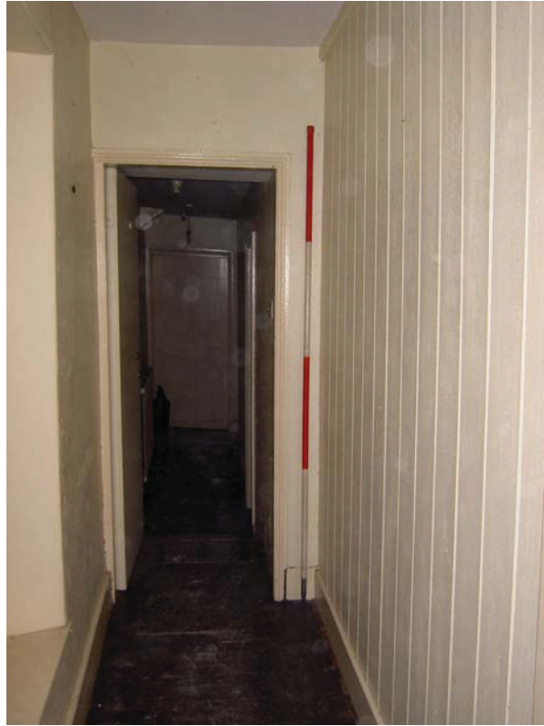
Plate 53: First floor Room 2 showing step in corridor and tongue and groove panelled partition wall
