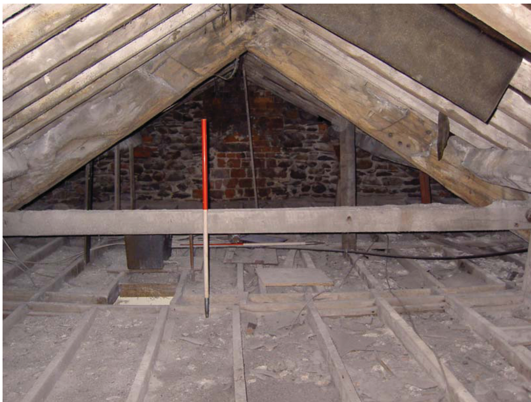
Plate 56: Detail of truss in roof space above first floor Rooms 8-10, showing re-used cruck blade fragments
