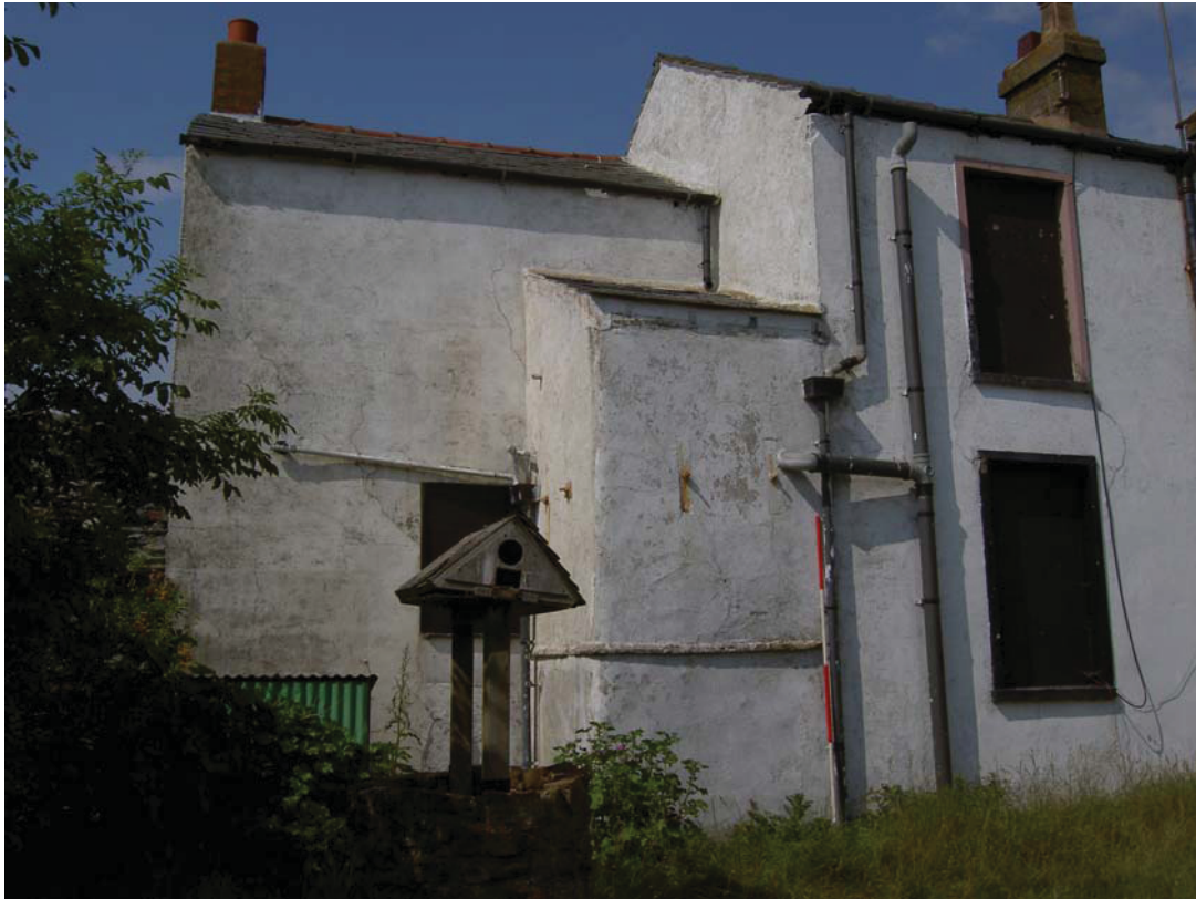
Plate 33: The west end of the south external elevation showing the tall outshut
