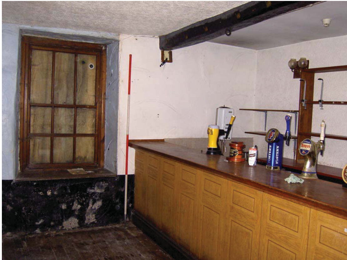
Plate 45: Bar, sliding sash window and stop chamfered beam in ground floor Room 8
